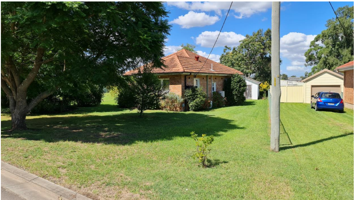
Below – Closer view of existing house being demolished along southern neighbour boundary.
