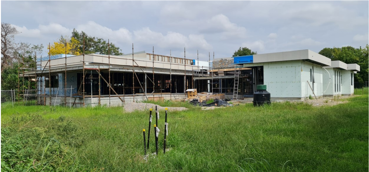
Rear view of dwelling under construction from the site for pool and pavilion/gym building.
