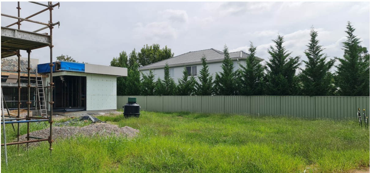
Further rear view of dwelling under construction and neighbouring two storey home.
