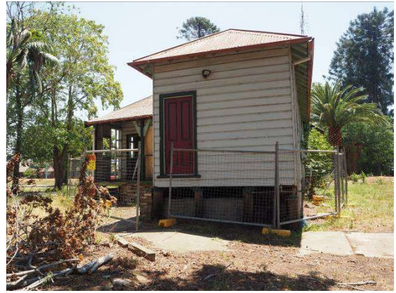
Figure 6: Southern (rear) elevation of former Police Station Building and location of proposed extension.
