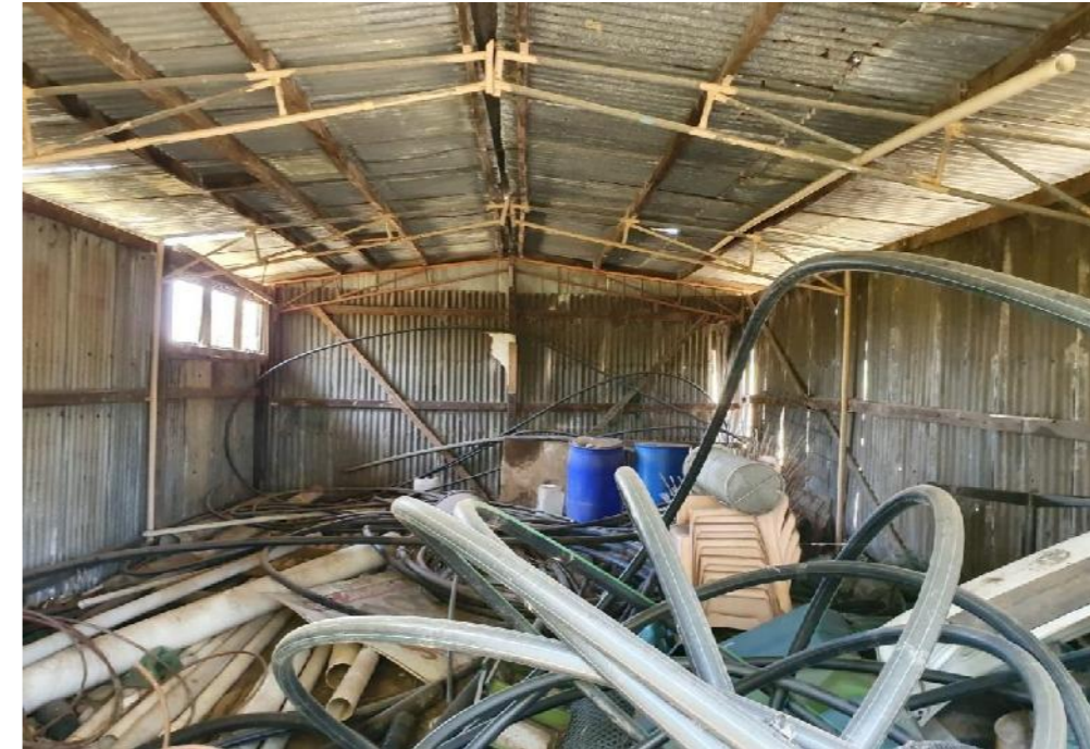
Photo 6 - Waste materials and drums stored in the easternmost shed
