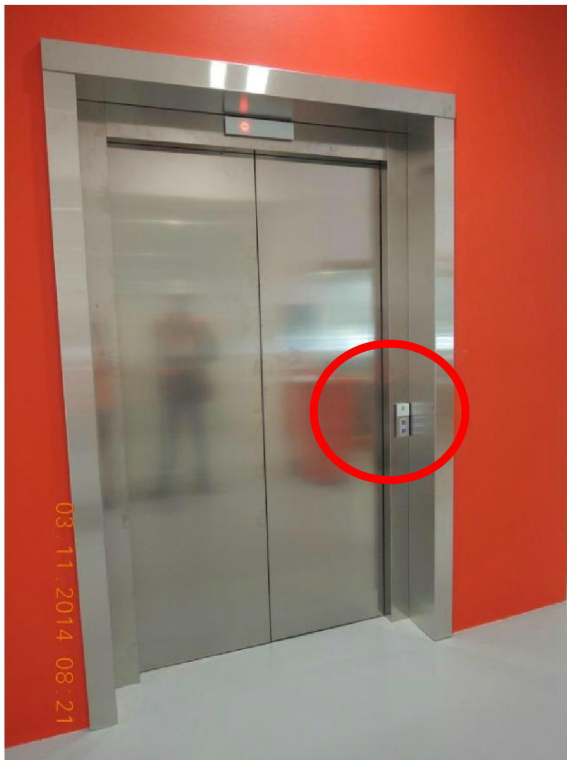
Figure 2 image of non-compliant lift call button installation
