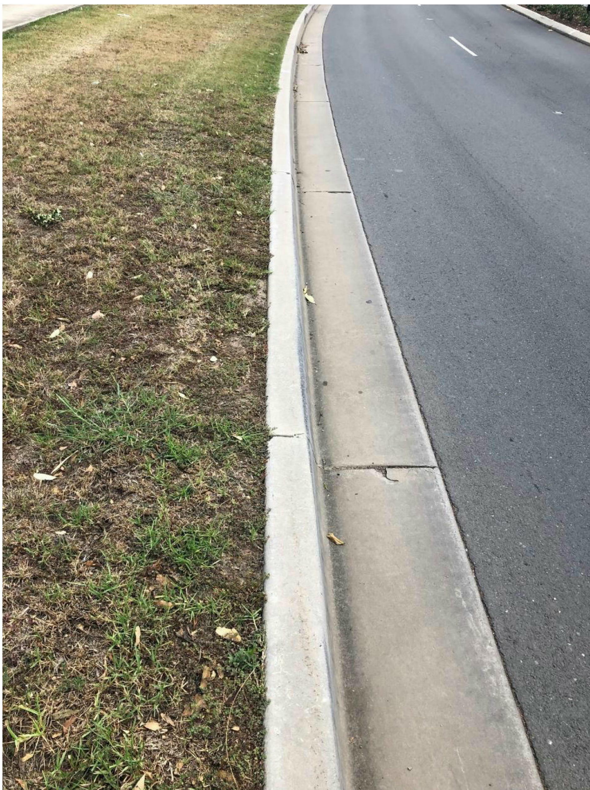
Figure 44: chip on construction joint interface on kerb and gutter.
