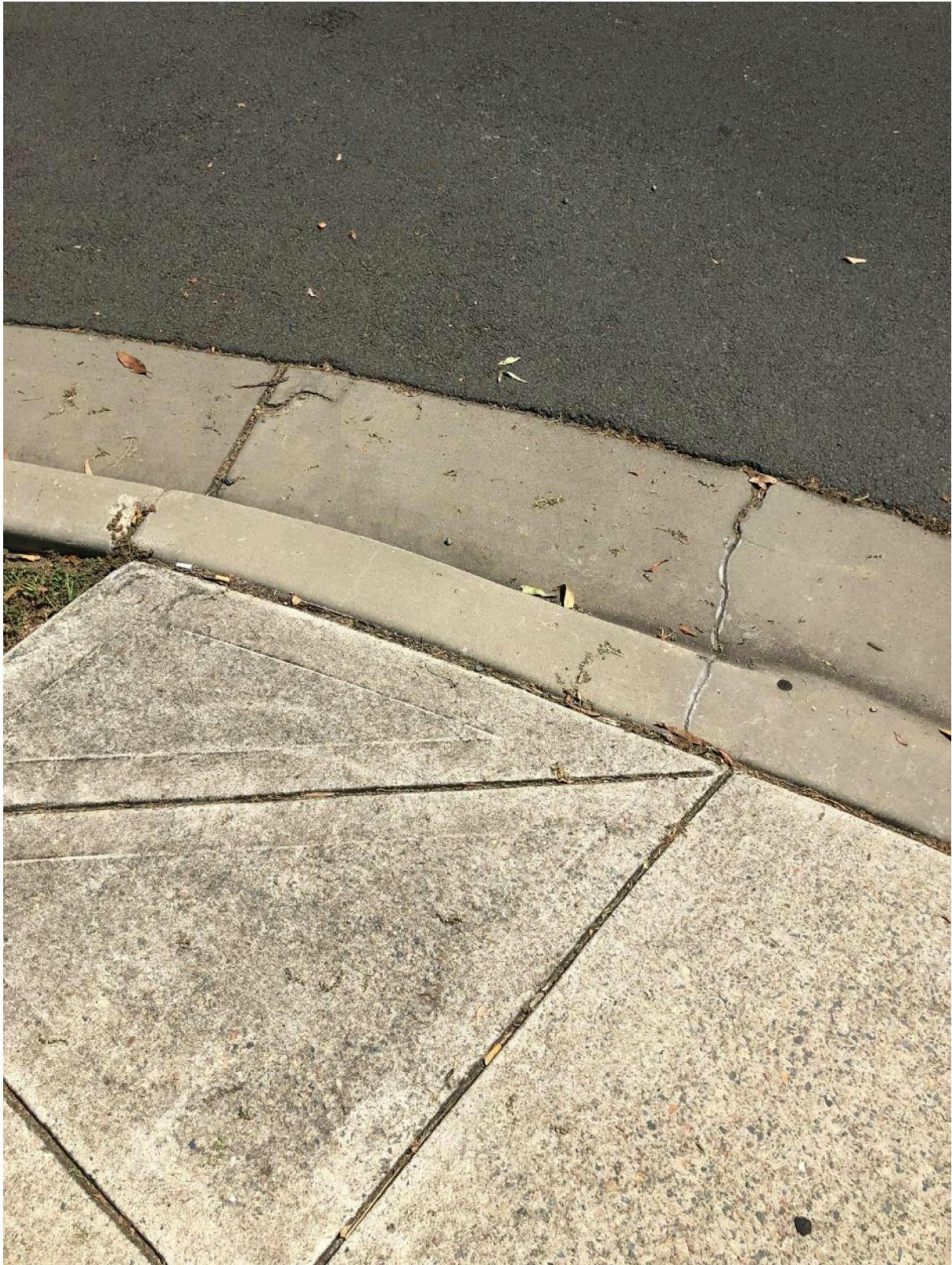
Figure 82: cracking to kerb and gutter, adjacent to right portion bottom of wing.
