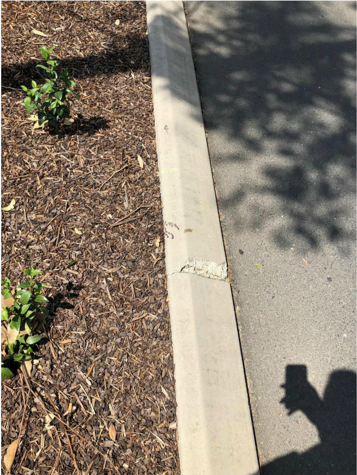
Figure 35: damage on construction joint interface.
