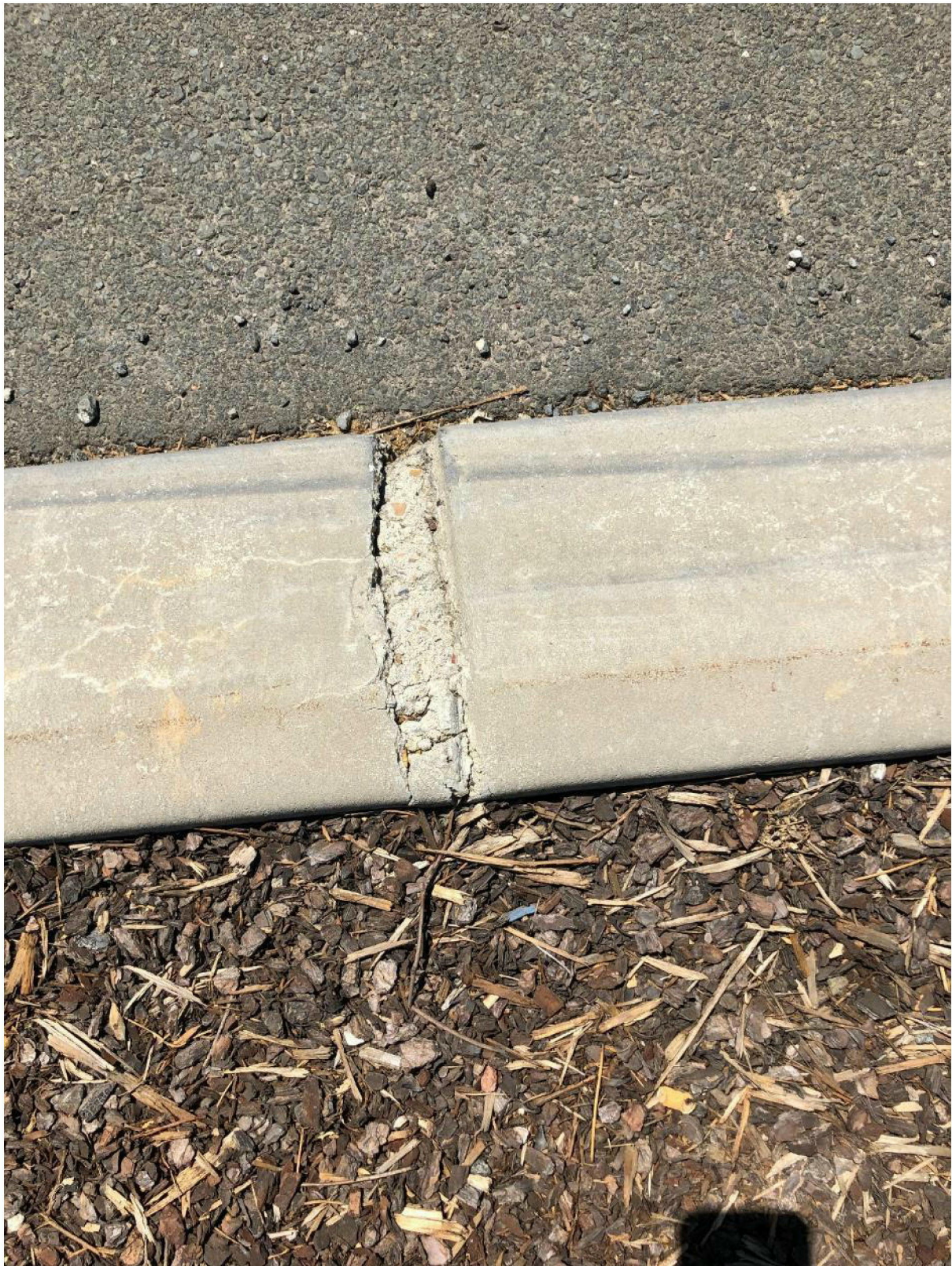
Figure 17: separation of kerb at construction joint interface.
