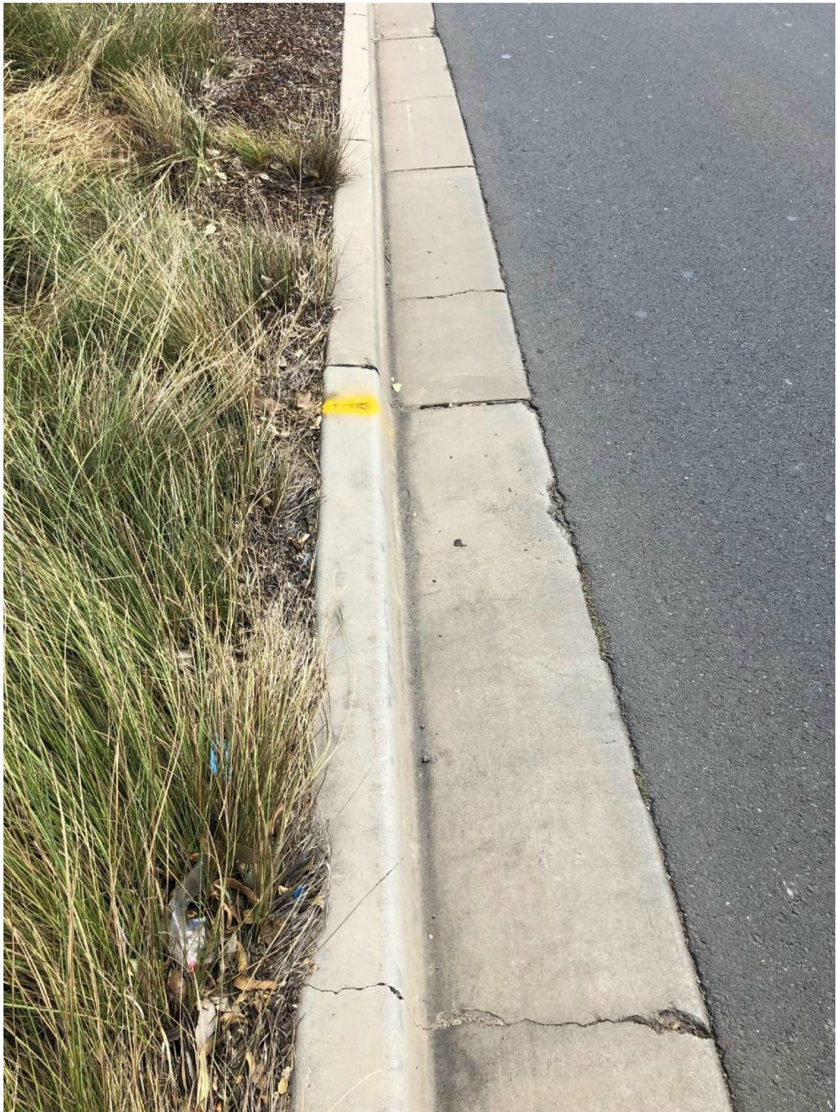
Figure 56: crack on kerb and gutter.
