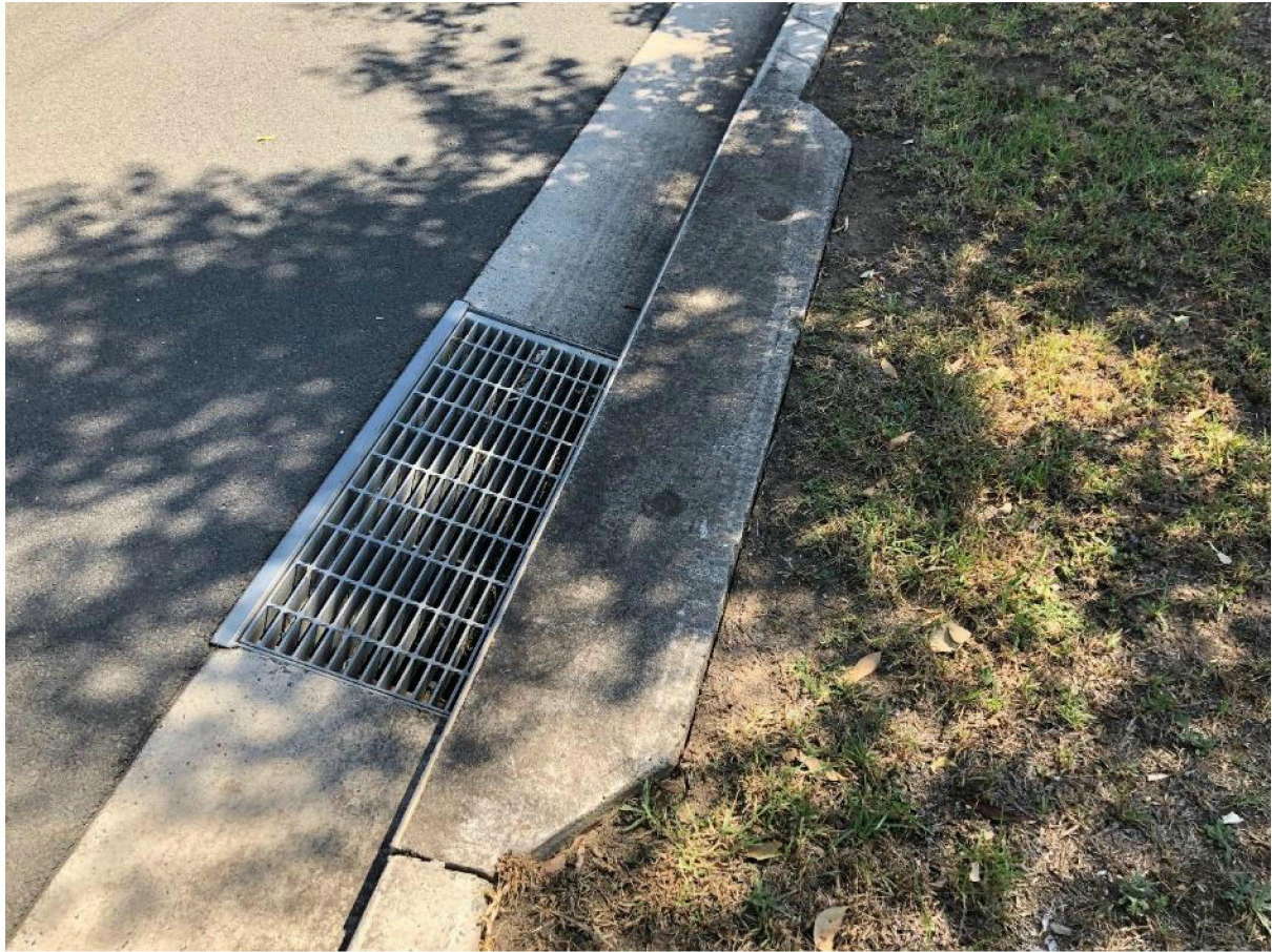
Figure 71: cracking to lintel and kerb joint (both sides).
