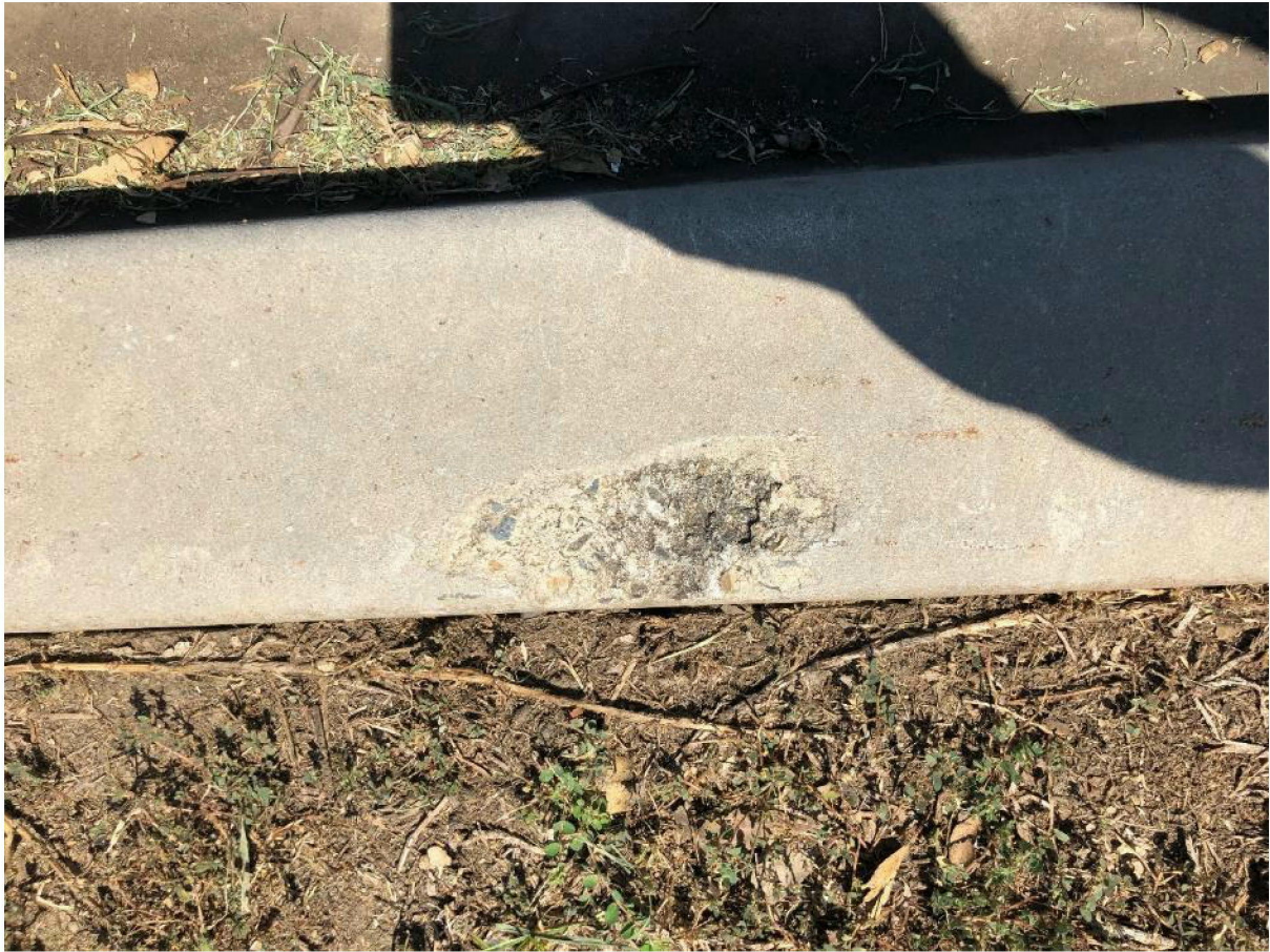
Figure 75: chip to top of gutter.
