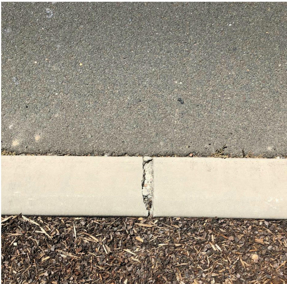
Figure 5: separation at construction joint interface.
