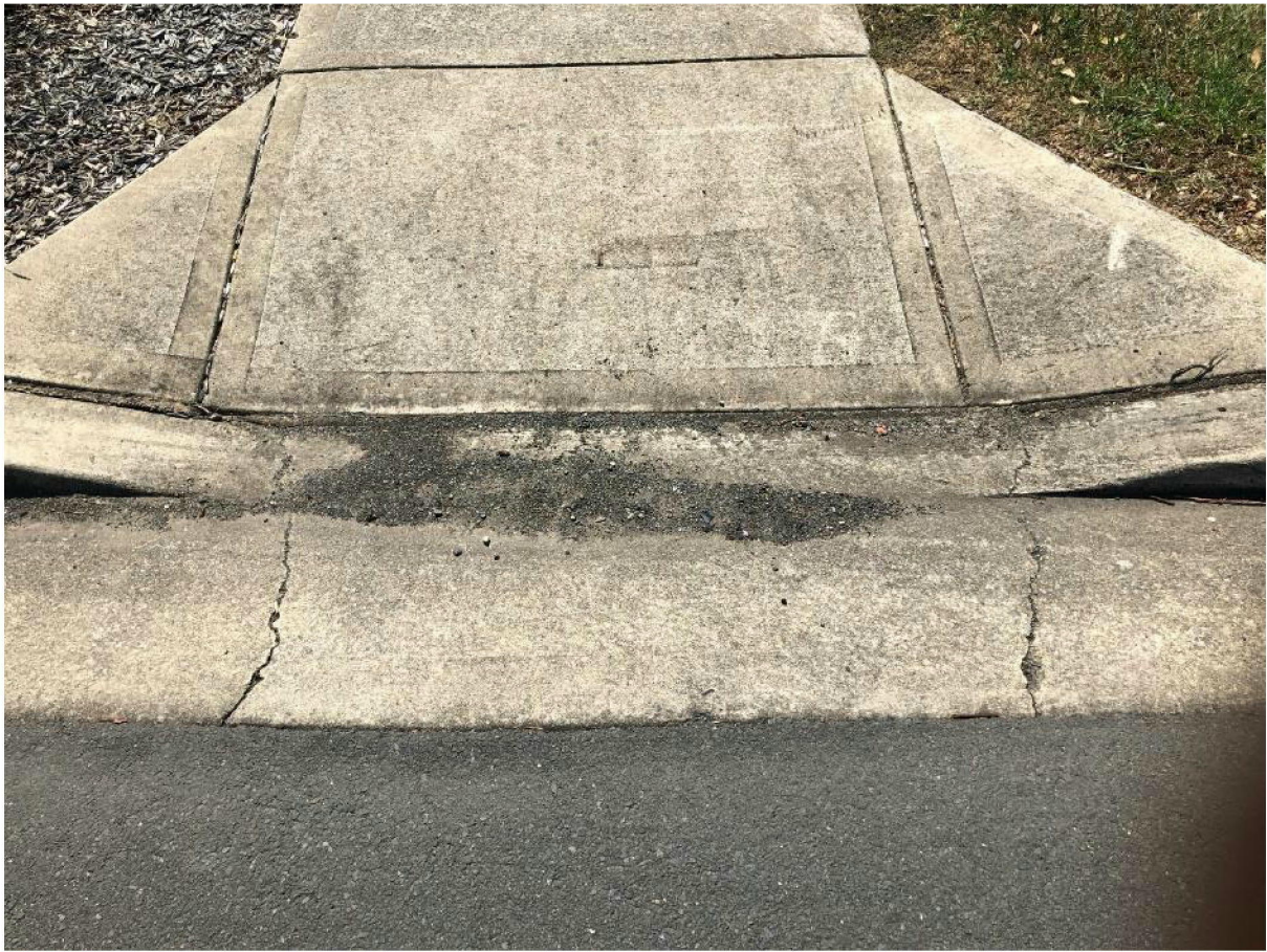
Figure 81: cracking to gutter, adjacent to flat portion of eastern pram ramp.
