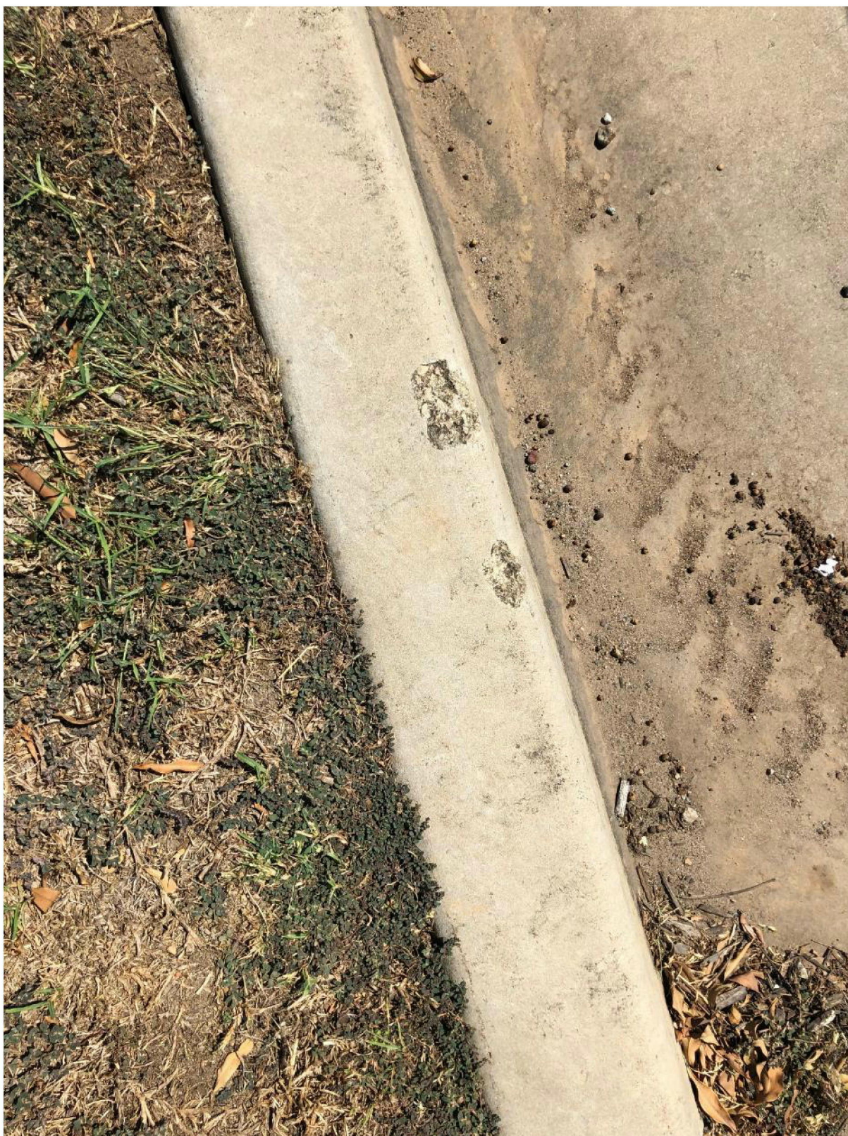
Figure 41: chips on top of kerb.
