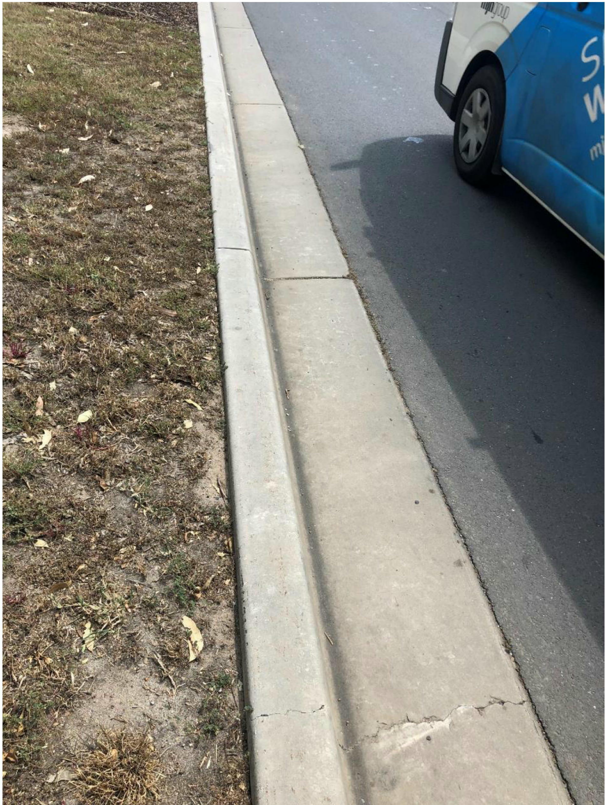
Figure 51: cracking to kerb and gutter.
