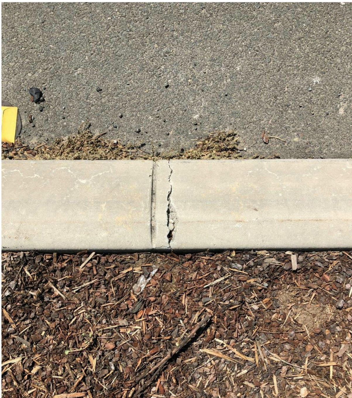
Figure 10: cracking to median strip, adjacent to construction joint.
