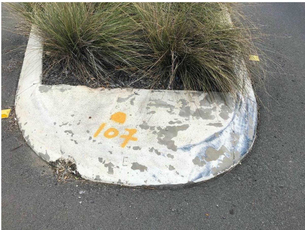
Figure 39: chip in median strip kerb (facing Lakeside Parade).
