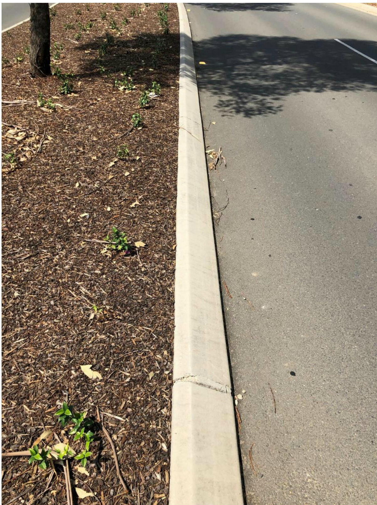
Figure 29: cracking on median strip kerb (adjacent to construction joint).
