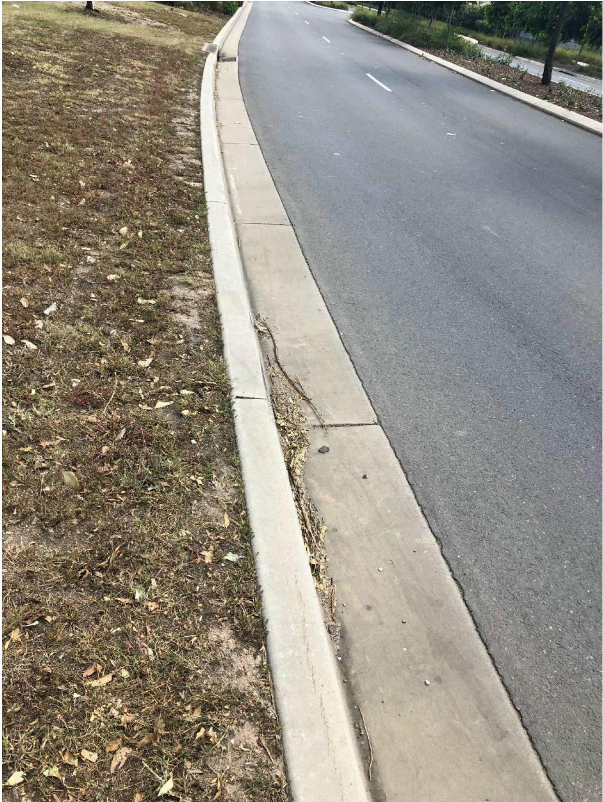
Figure 47: indentation to concrete gutter.
