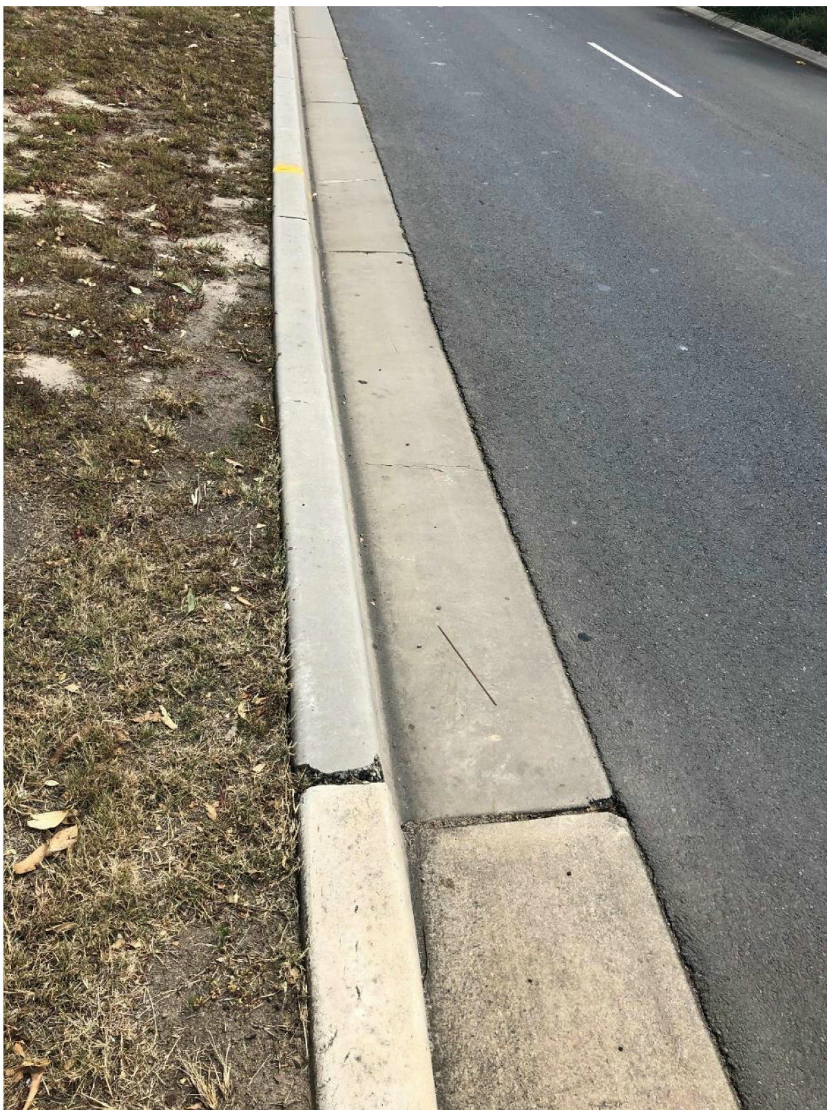
Figure 50: damage to expansion joint interface on kerb and gutter.
