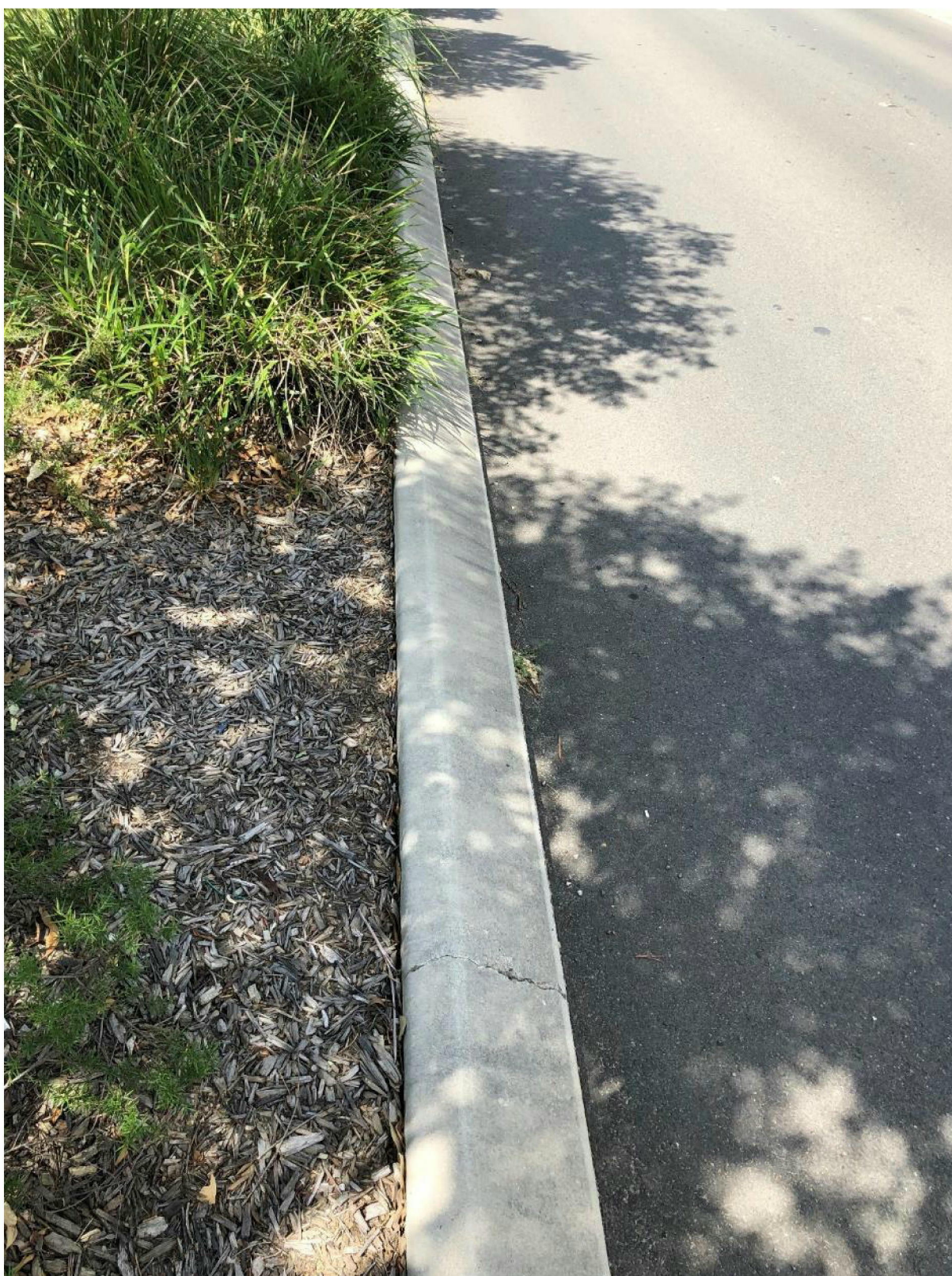
Figure 27: cracking to median strip kerb.
