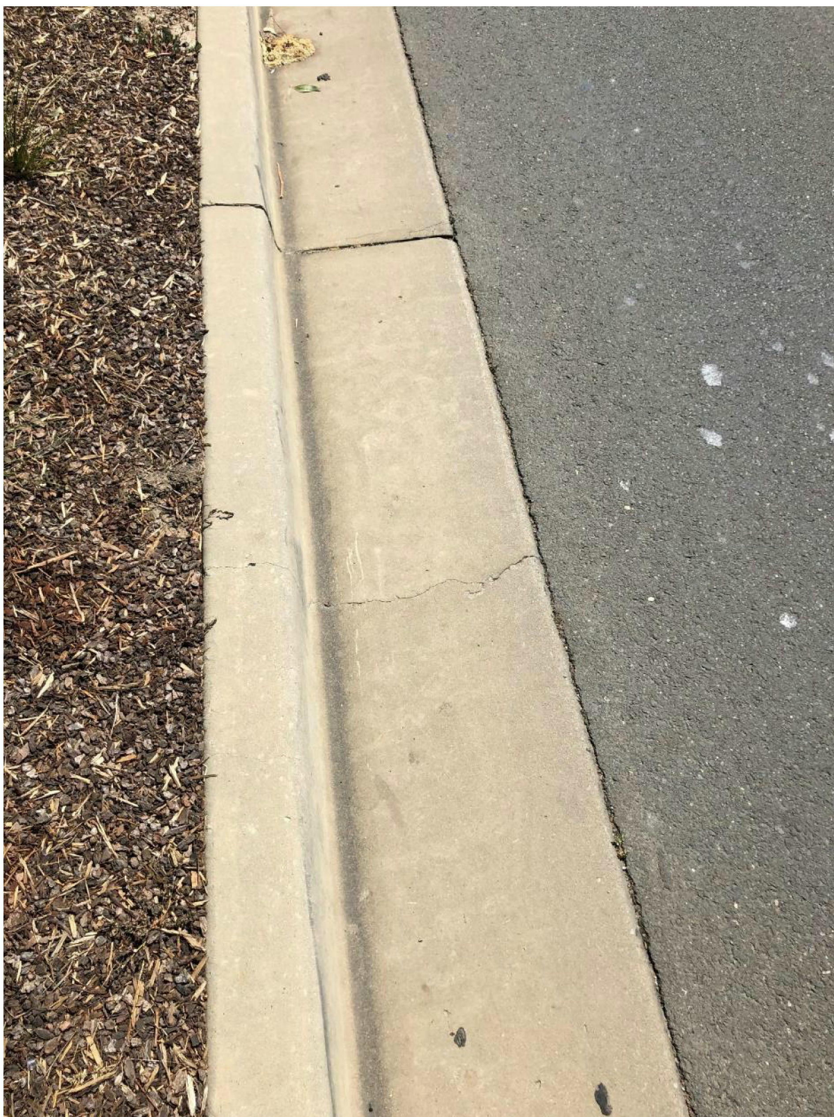
Figure 60: cracking to kerb and gutter.
