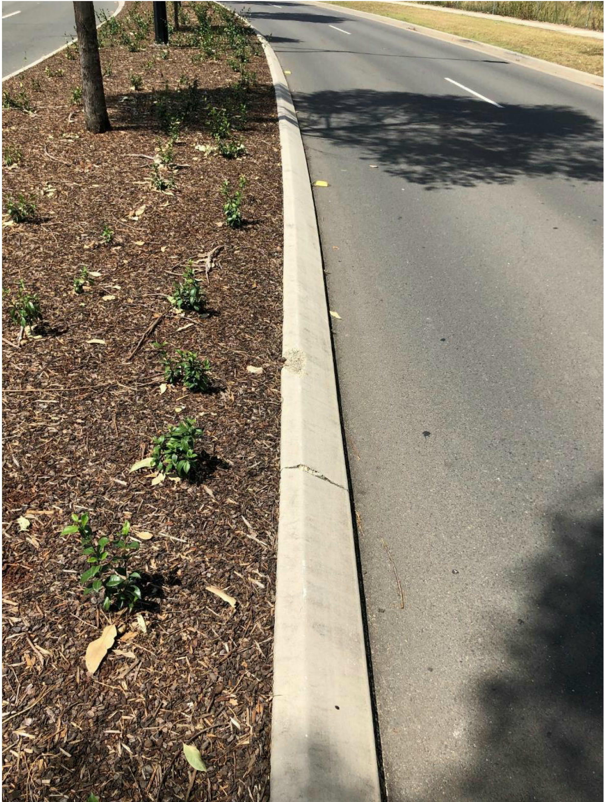
Figure 30: damage on construction joint interface.
