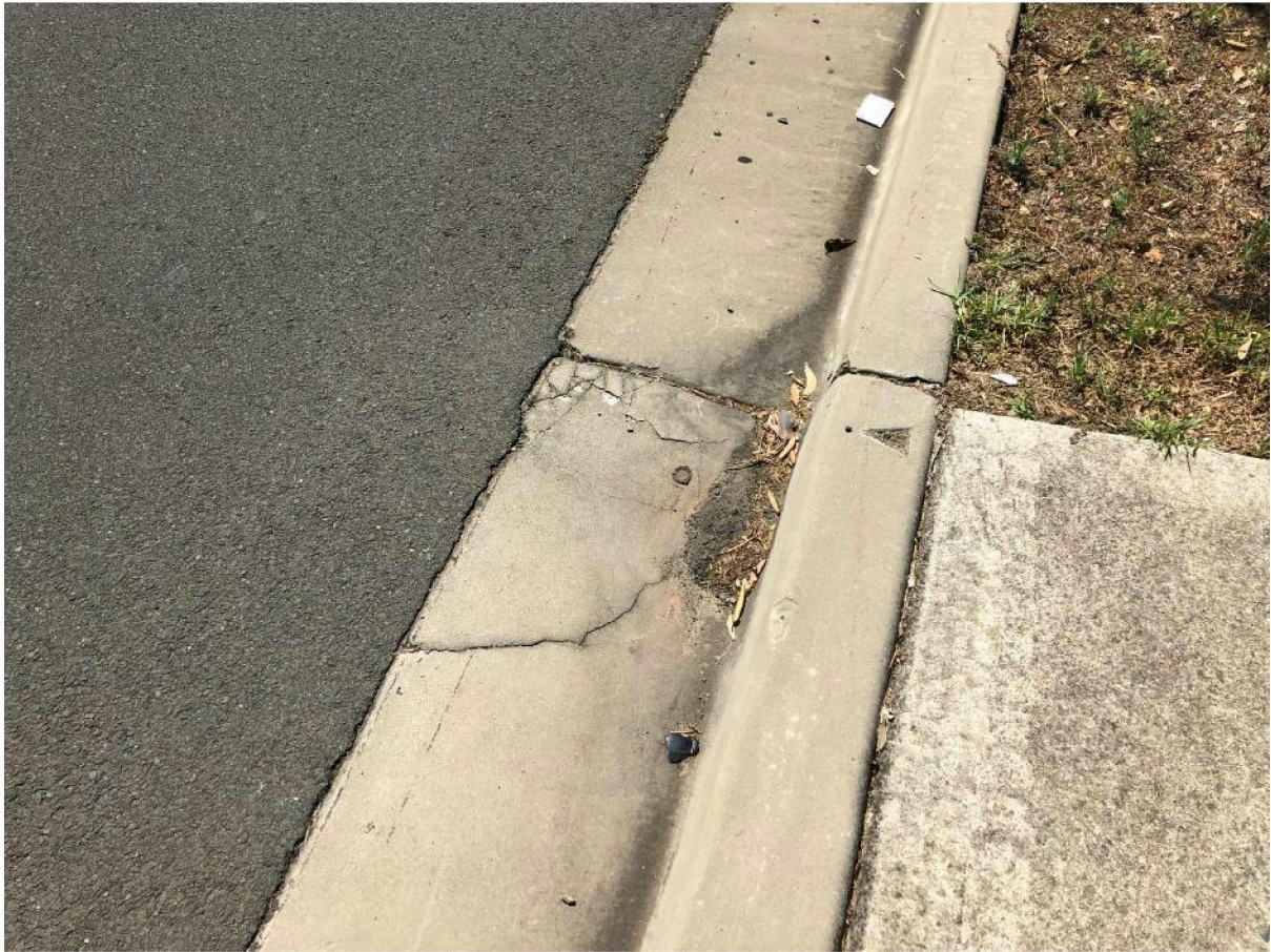
Figure 83: cracking to gutter, adjacent to top of left wing.
