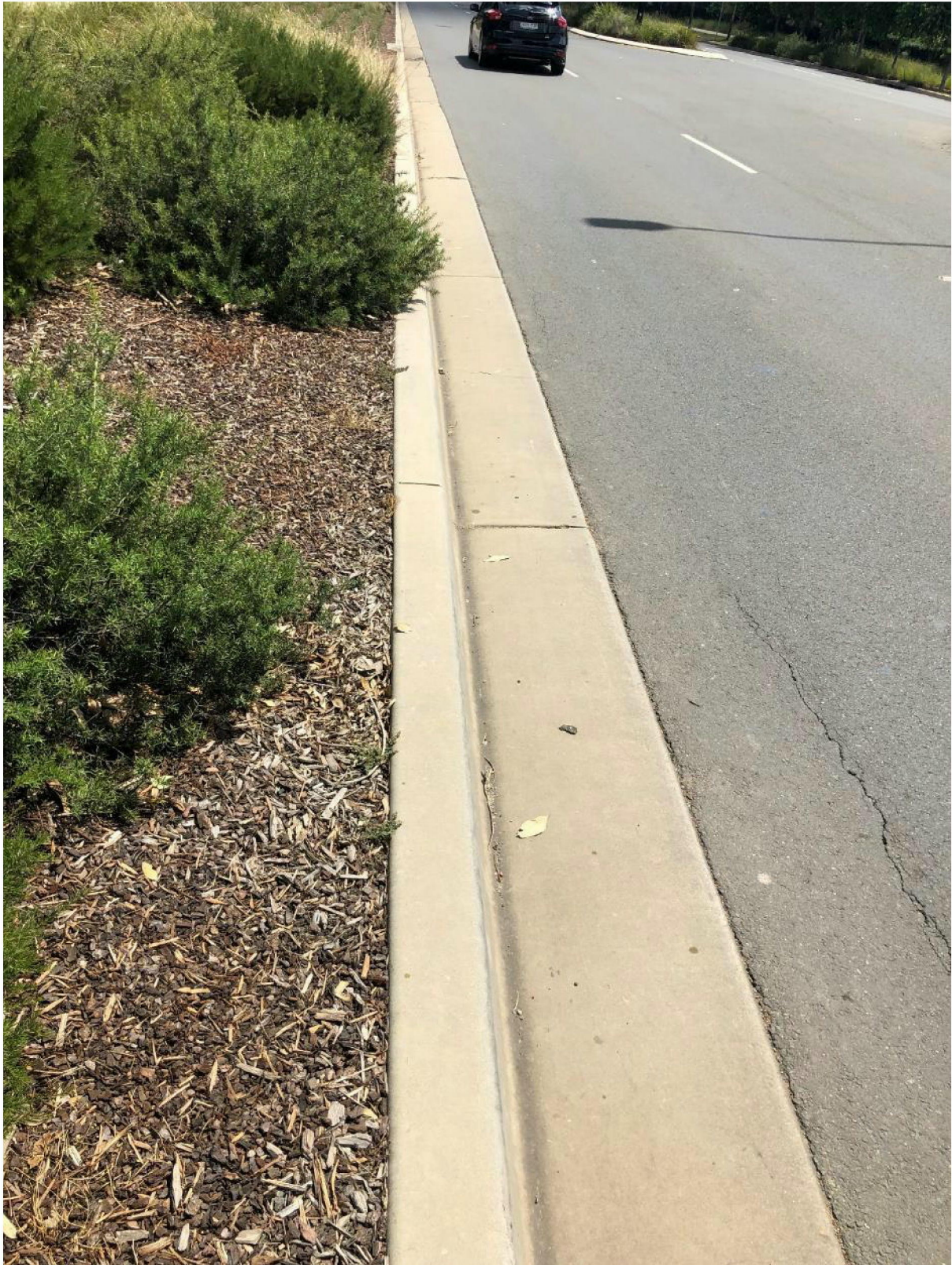
Figure 54: crack on asphalt, adjacent to gutter.
