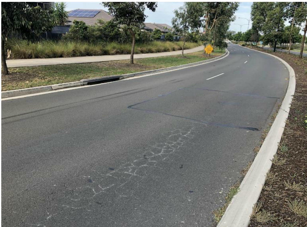
Figure 89: Approx CH255 EB Pavement failure
