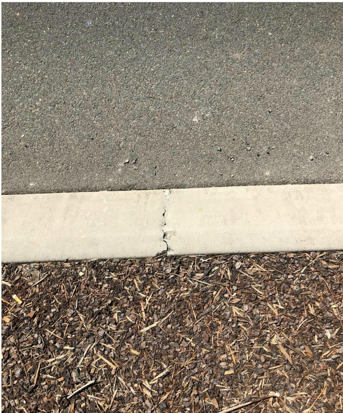
Figure 7: cracking to median strip kerb.
