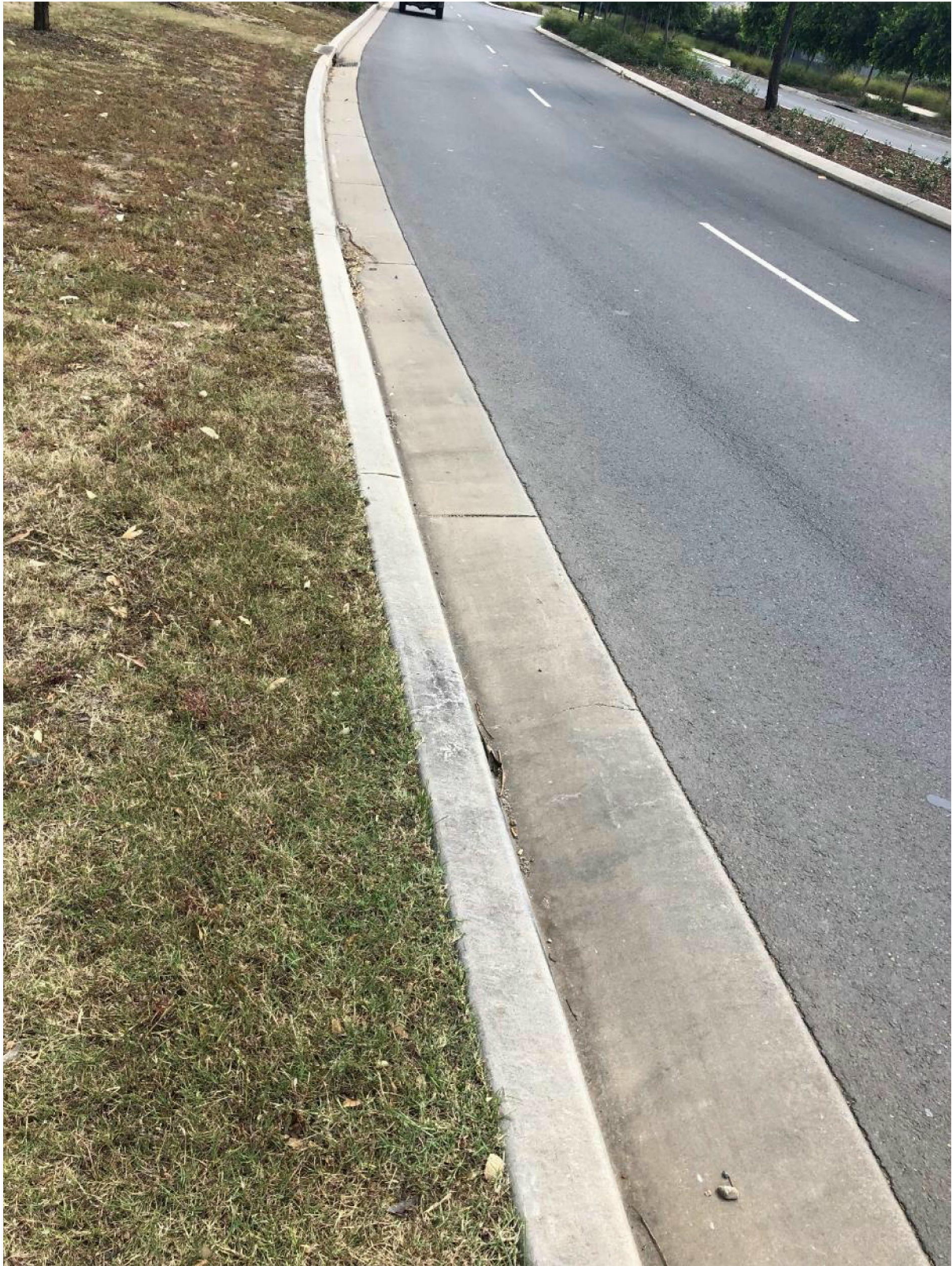
Figure 46: minor cracking to gutter.
