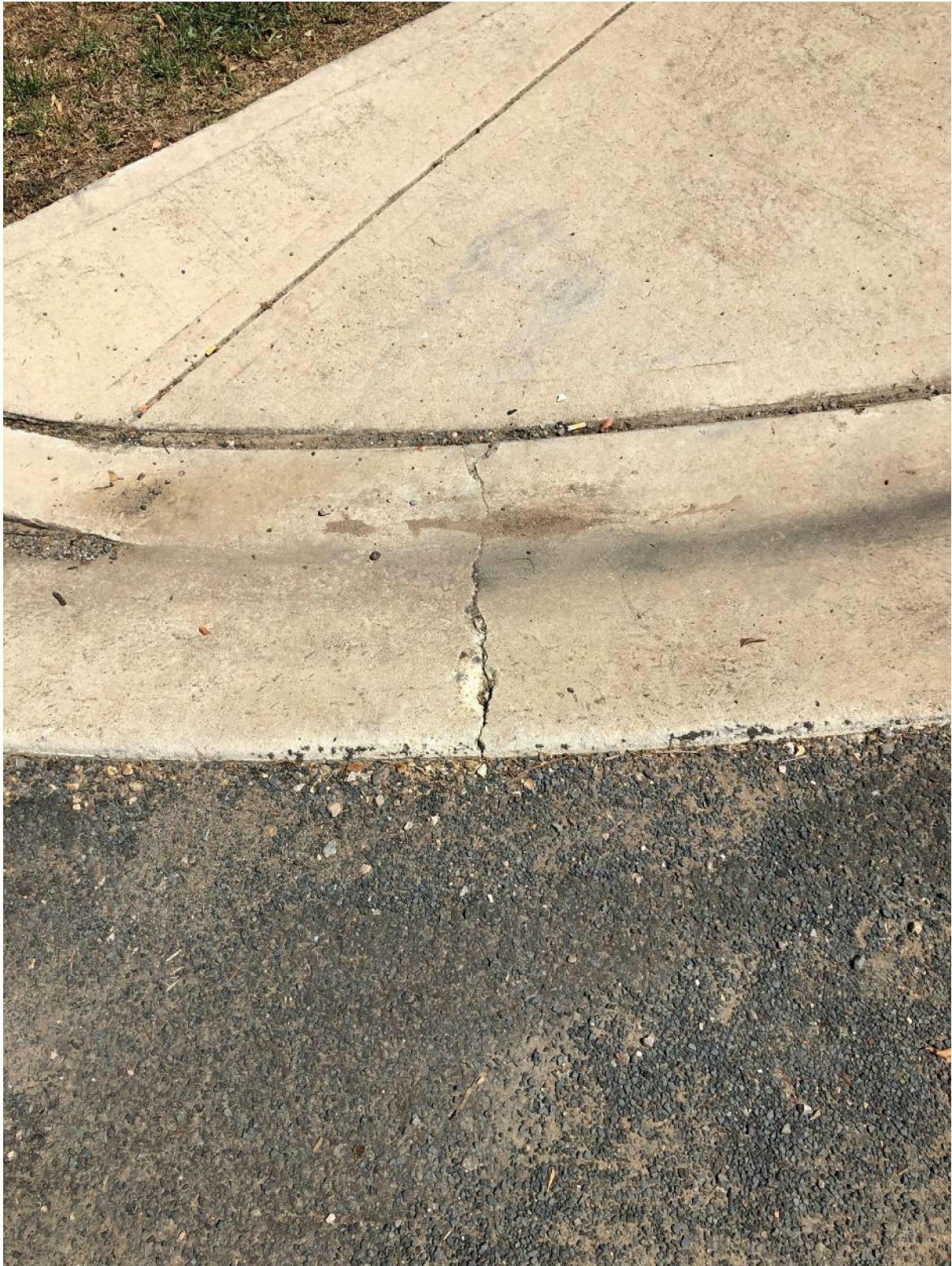
Figure 86: cracking to gutter, adjacent to pram ramp located right of proposed site entry.
