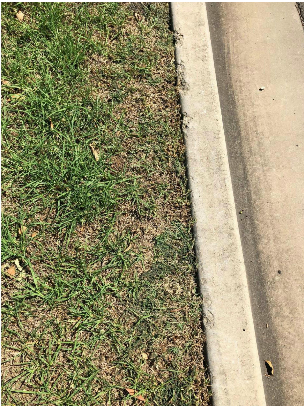
Figure 40: chips to top of kerb and gutter.
