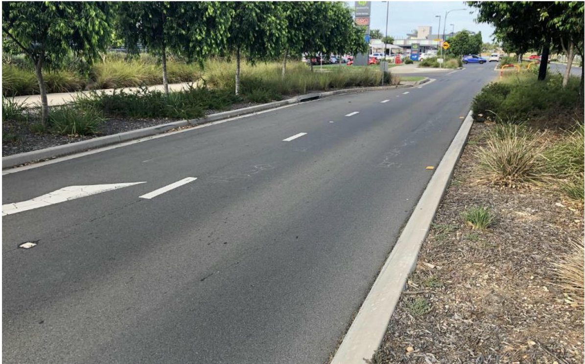
Figure 90: CH325-330 Pavement failure at wheel track (P70)
