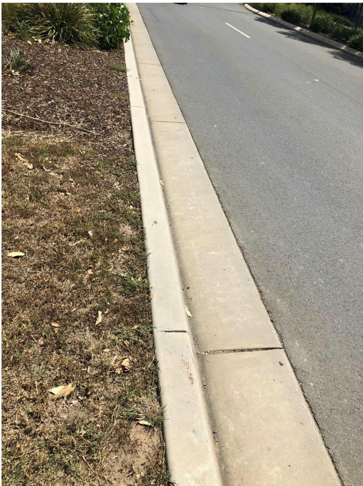
Figure 52: cracking to top of kerb.
