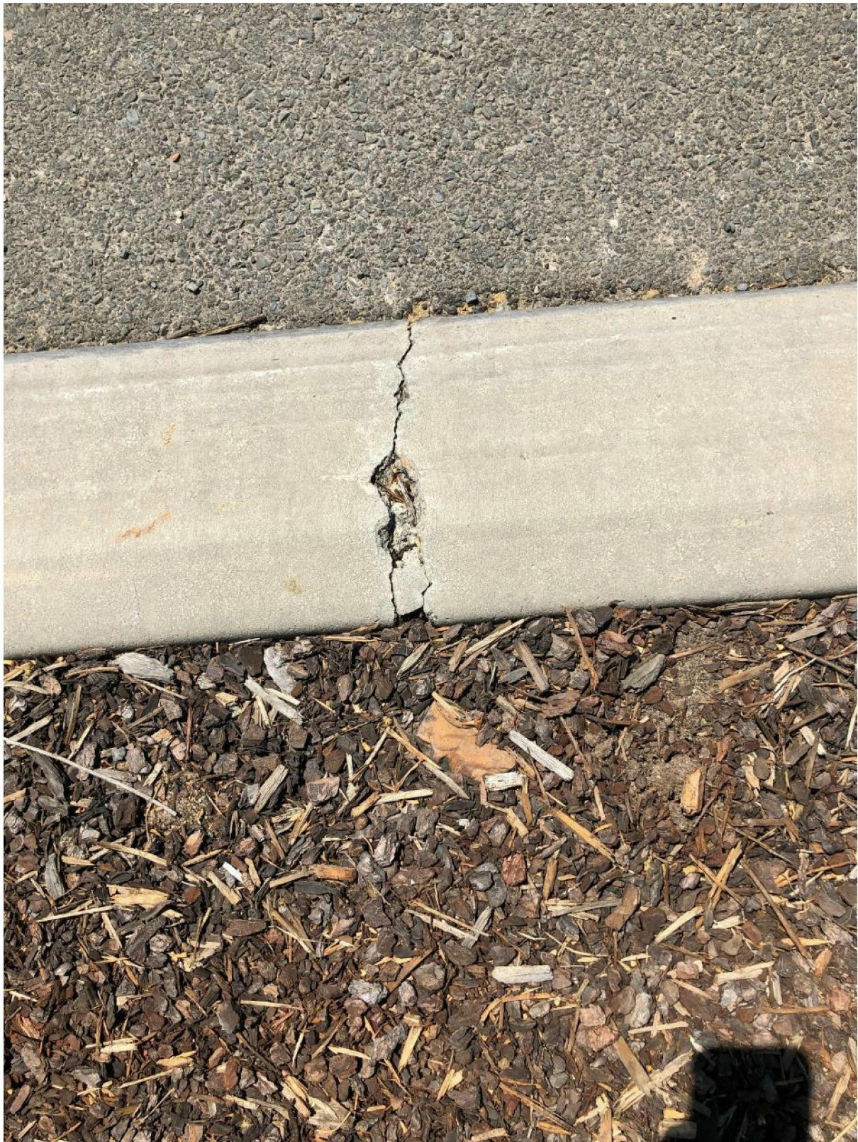
Figure 15: cracking to median strip kerb.
