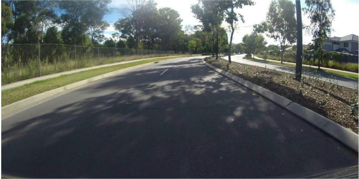
Figure 94: Approx CH200 WB horizontal crack
