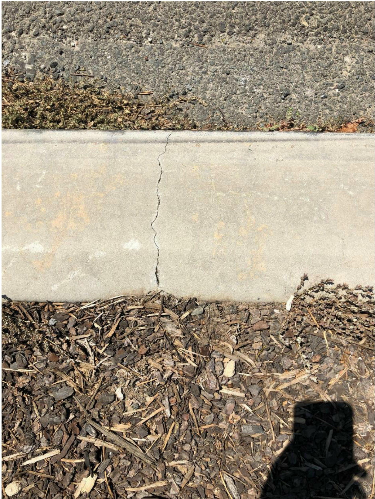
Figure 12: cracking to median strip kerb.
