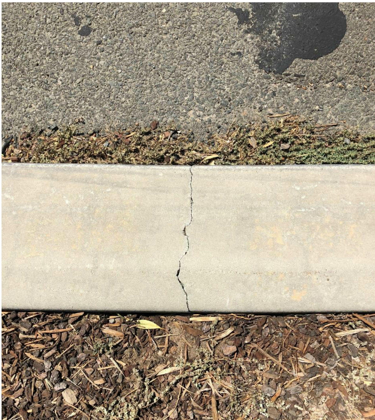
Figure 11: cracking to median strip kerb.
