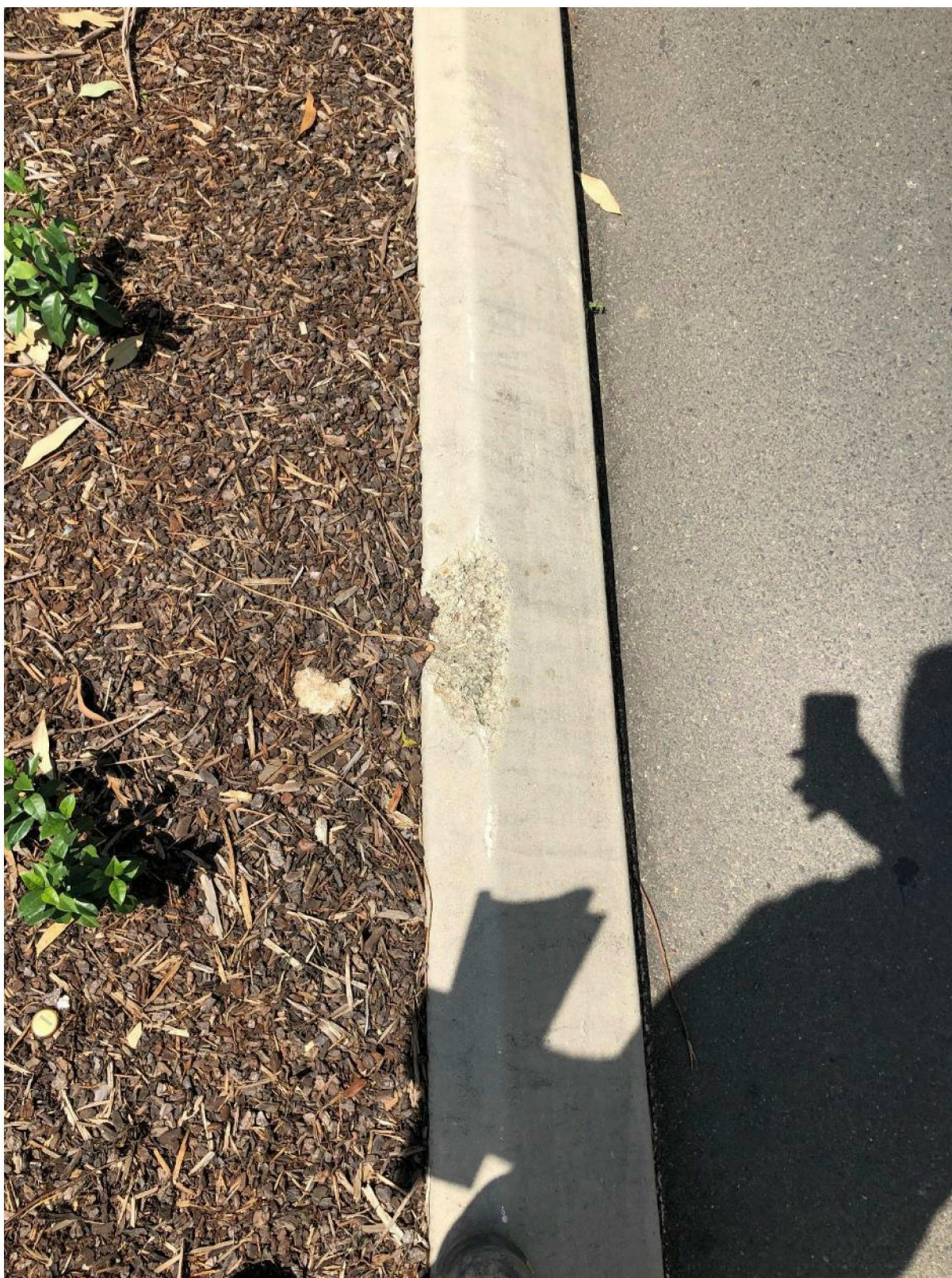
Figure 31: chip on top of median strip kerb.
