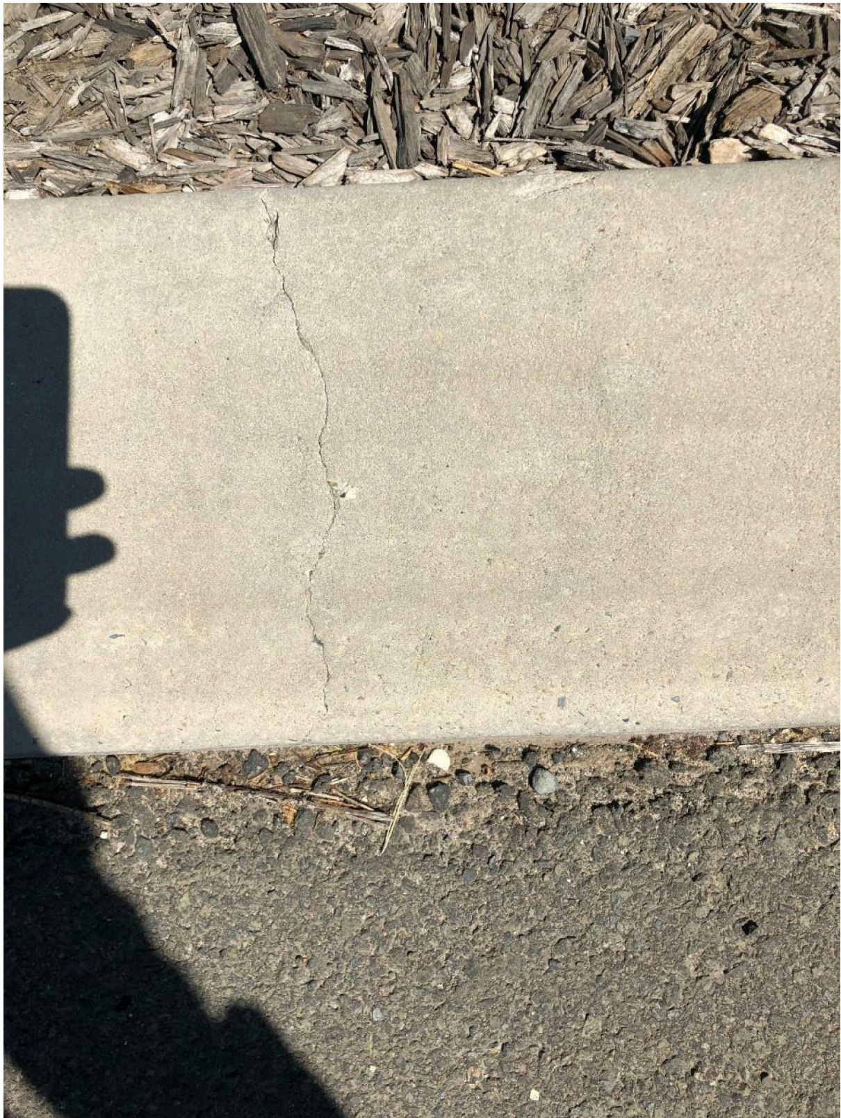
Figure 2: crack in median strip kerb.
