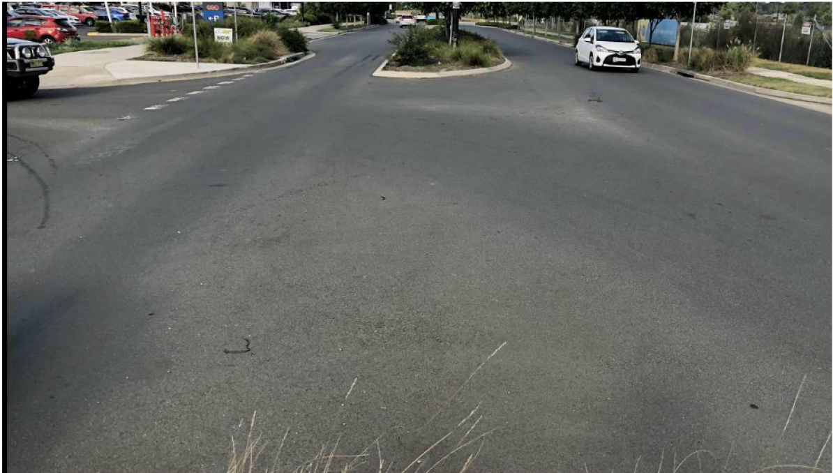
Figure 92: CH475 EB pavement failure at McGarrity Pde (P78)
