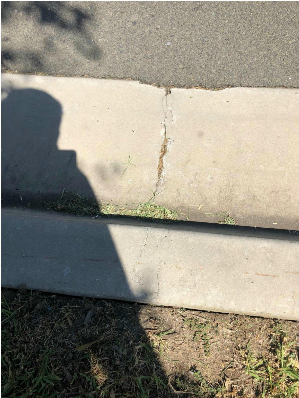
Figure 73: cracking to gutter and top of kerb.
