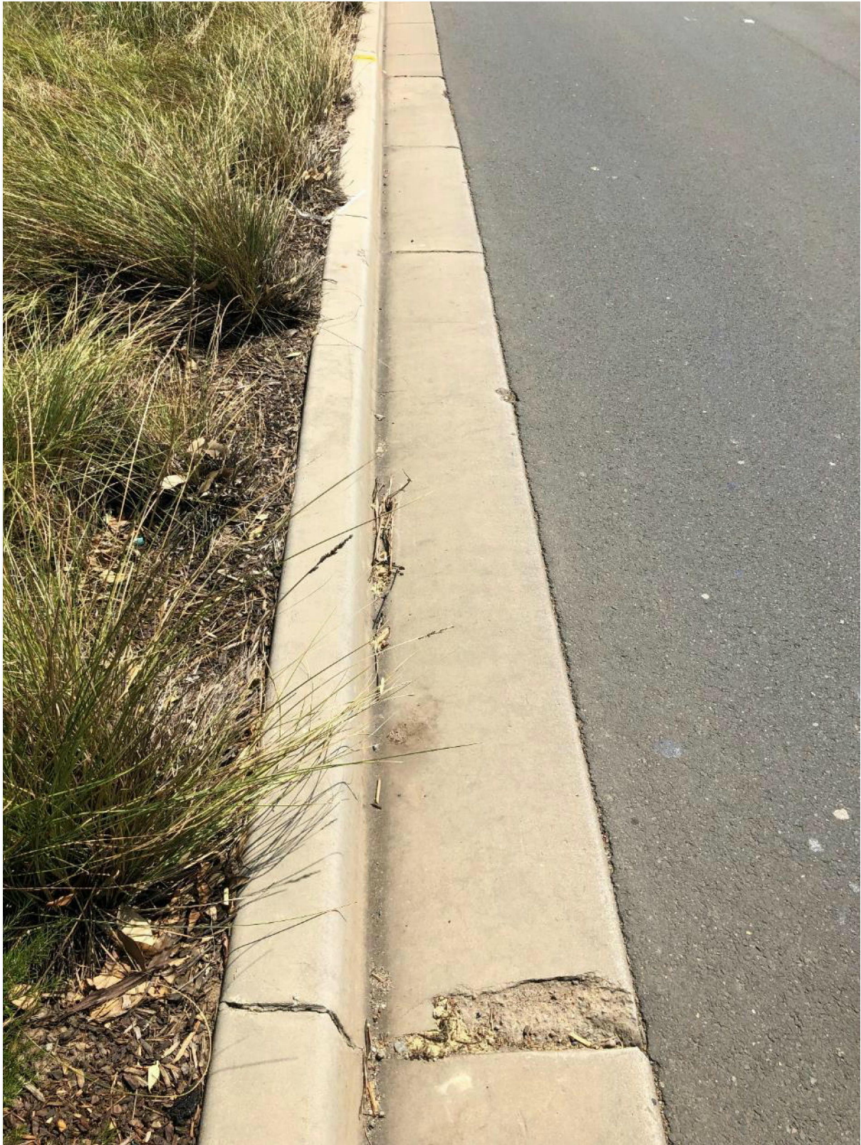
Figure 55: spalling to gutter, expansion joint interface.
