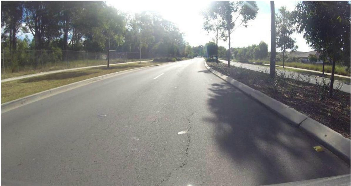
Figure 96: CH250 WB pavement crack/failure
