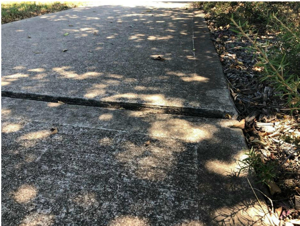
Figure 84: footpath bay lifted at expansion joint interface.
