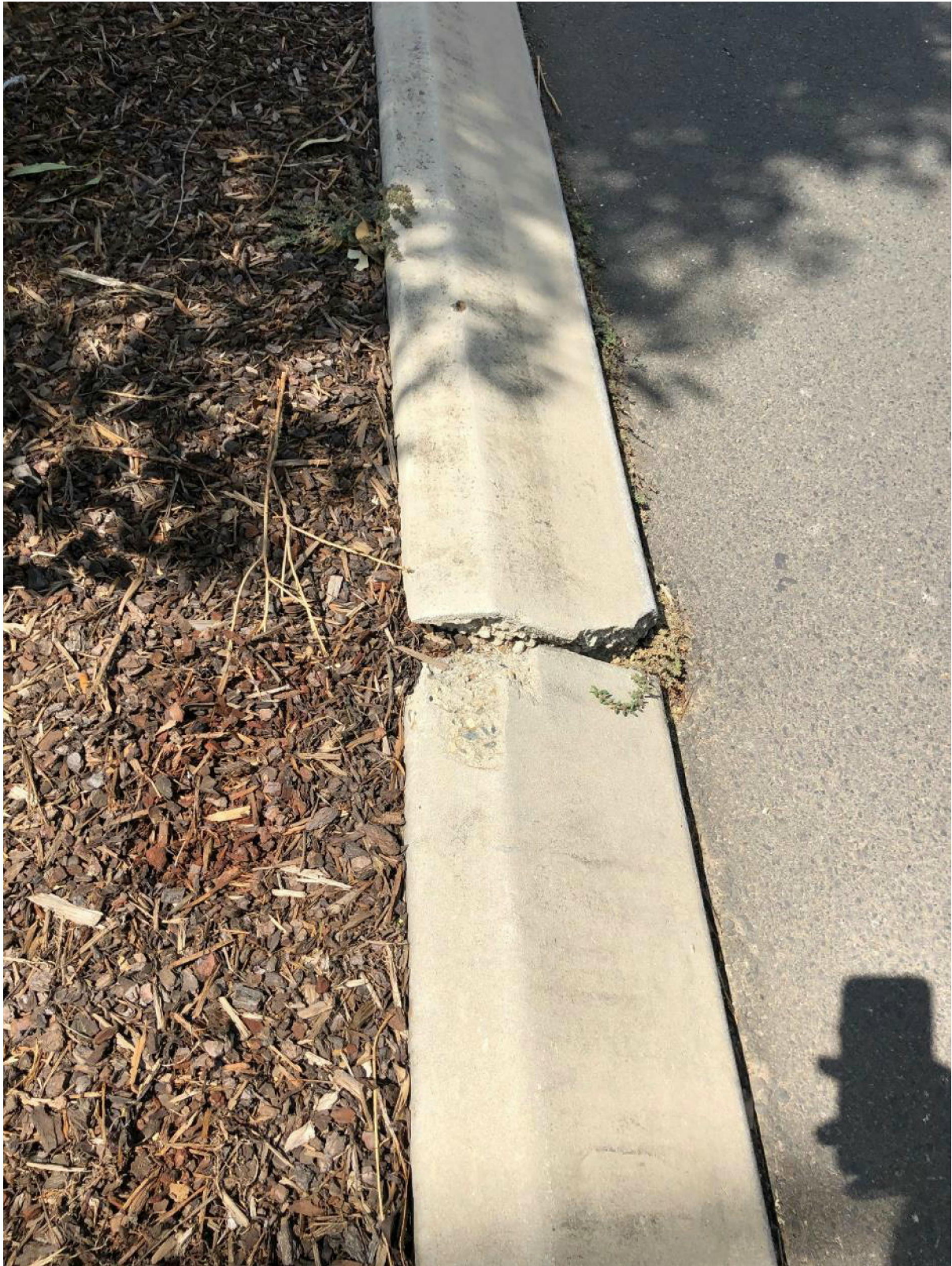
Figure 33: separation at construction joint interface.
