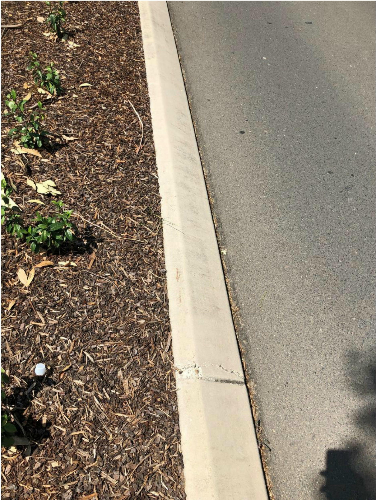
Figure 36: spalling on construction joint interface.
