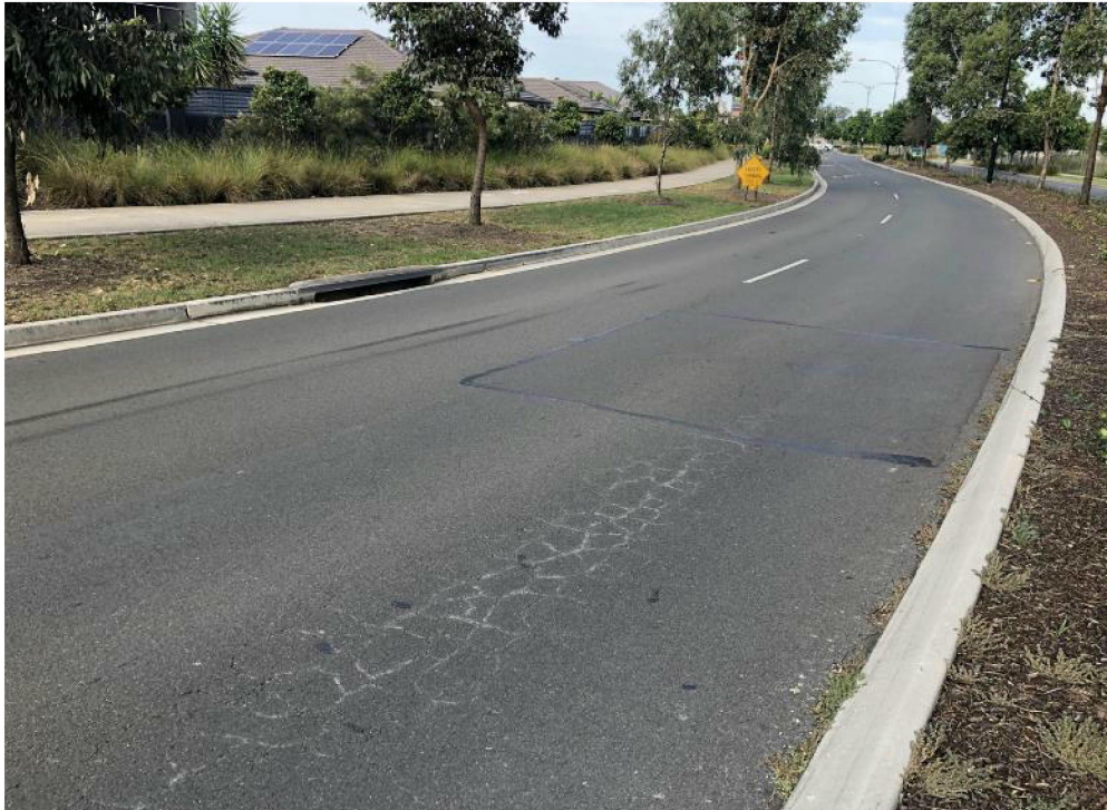
Figure 89: Approx CH255 EB Pavement failure
