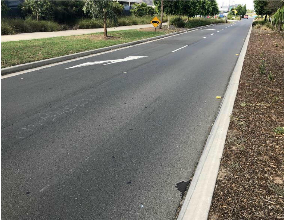
Figure 90: Approx CH300 EB Pavement failure (P66)
