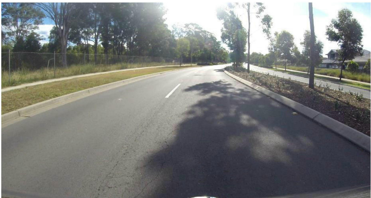
Figure 95: Approx CH210 WB Pavement failure
