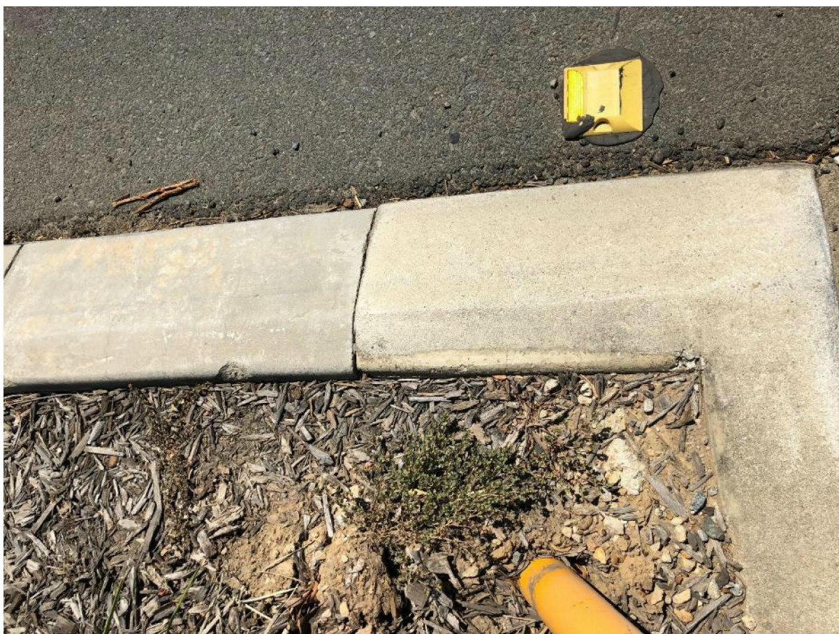
Figure 26: chips to top of median strip kerb.
