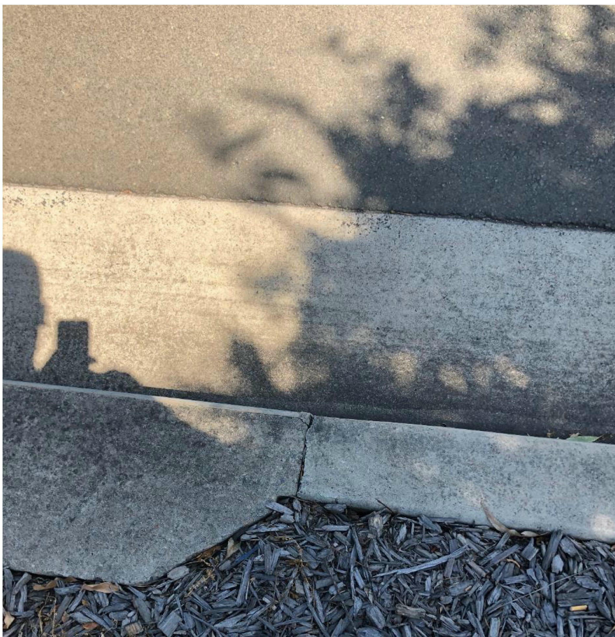
Figure 64: cracking at lintel and kerb joint (both sides of lintel).
