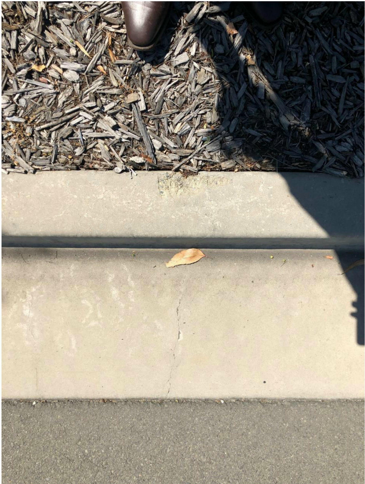
Figure 63: chip on top of kerb and minor cracking on gutter.
