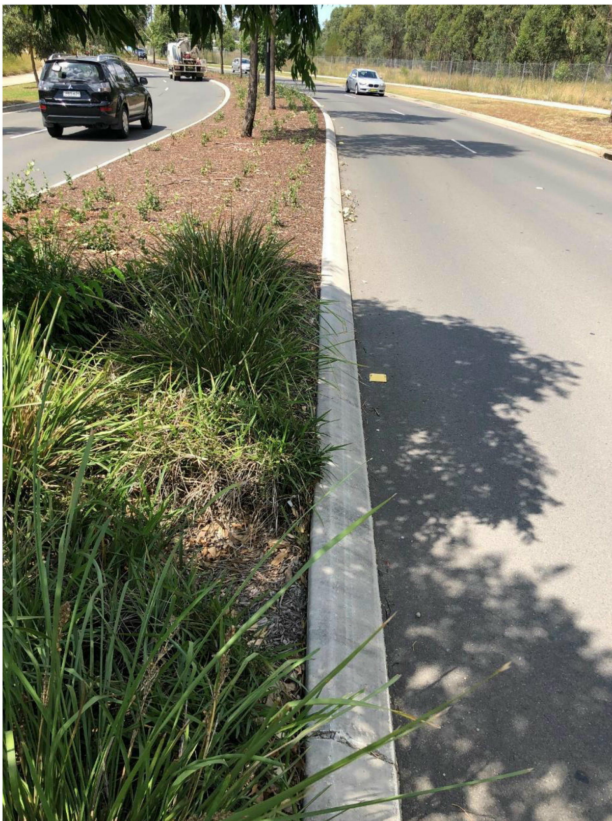
Figure 28: damage at joint interface of median strip kerb.
