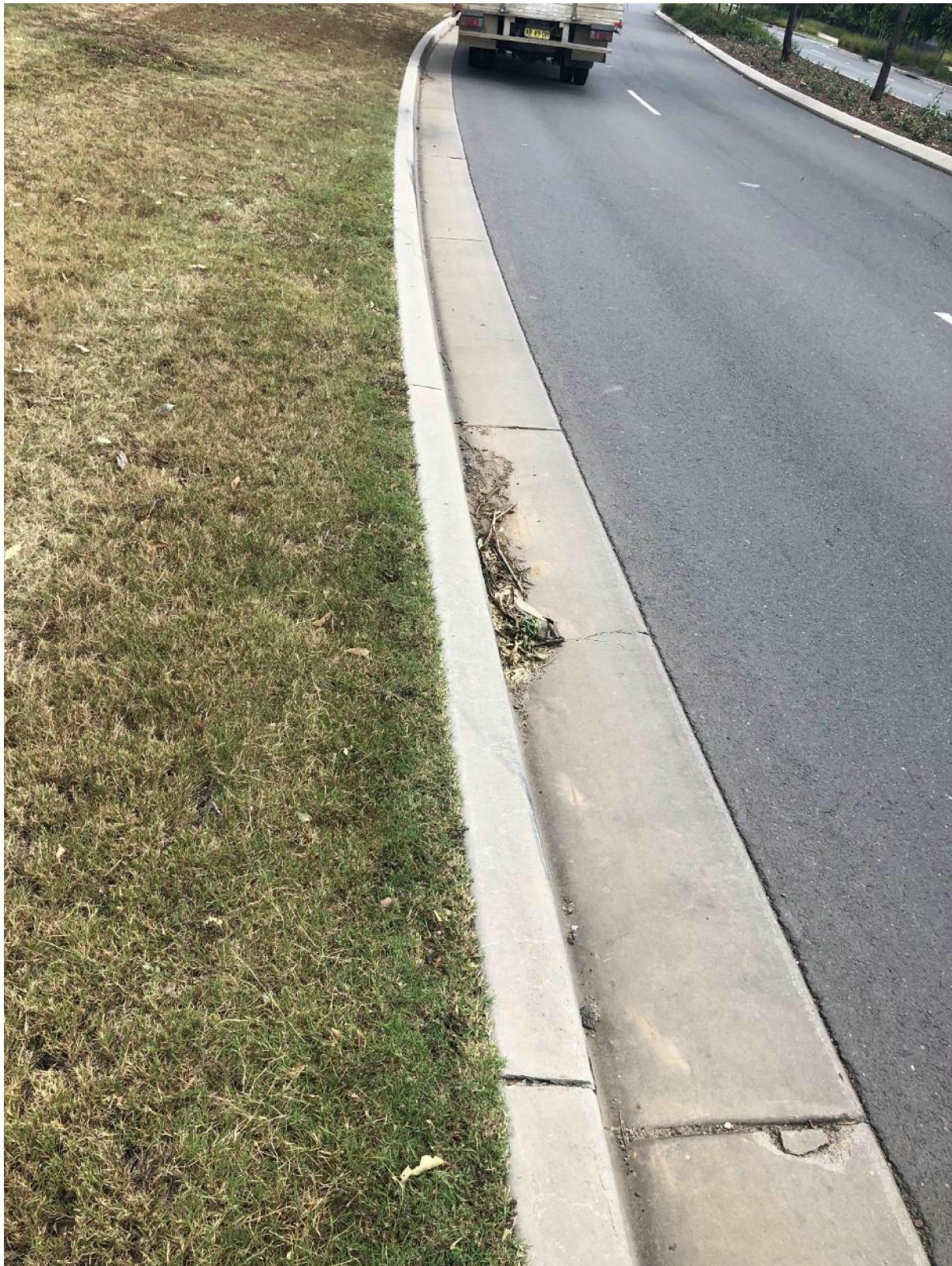
Figure 45: chip damage to kerb & gutter construction joint interface and cracking.
