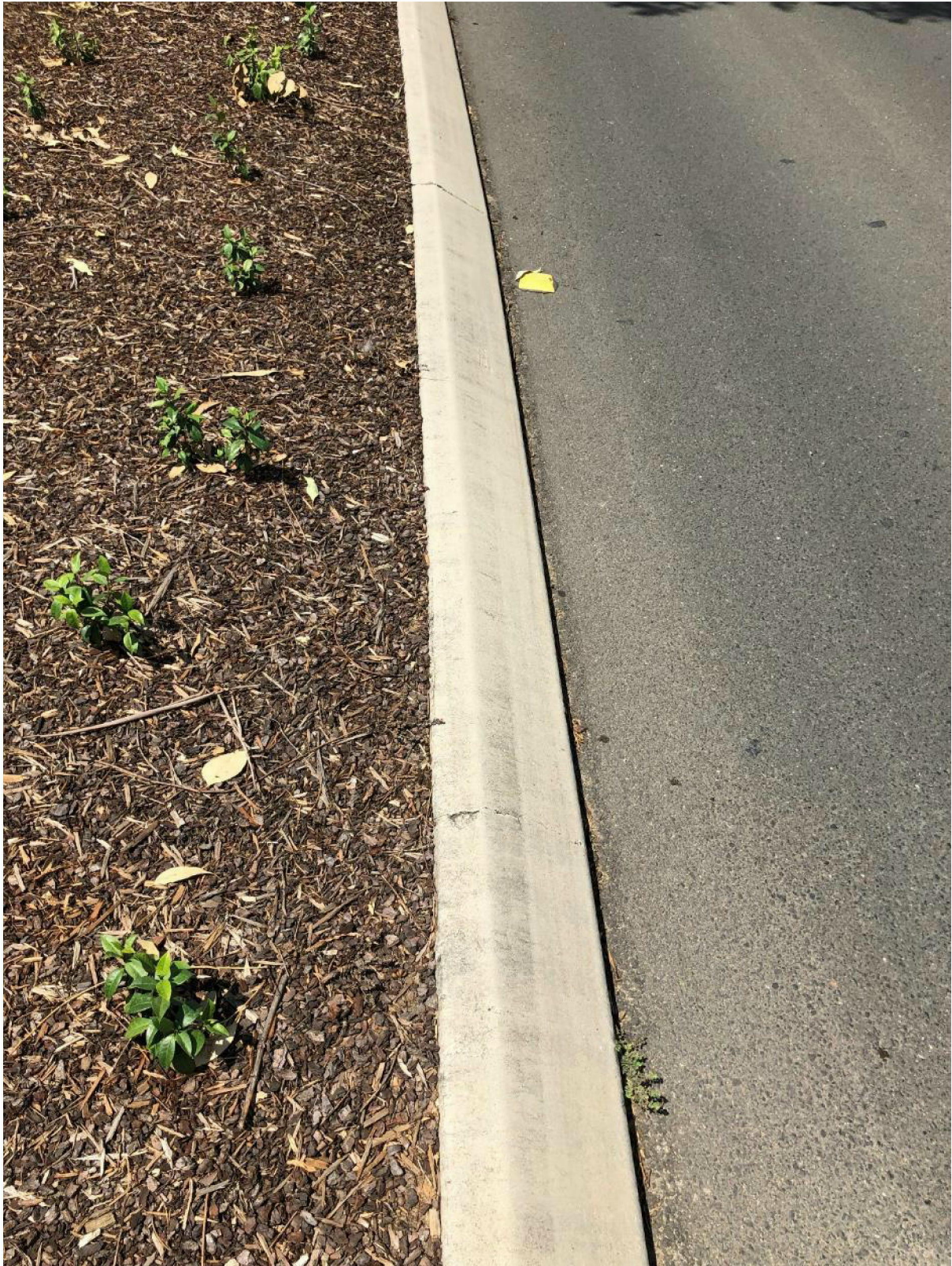
Figure 34: cracking to median strip kerb.
