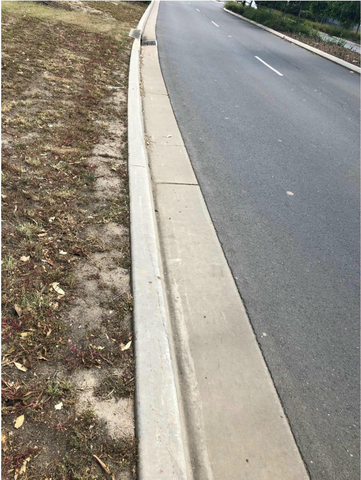
Figure 48: crack on concrete gutter.
