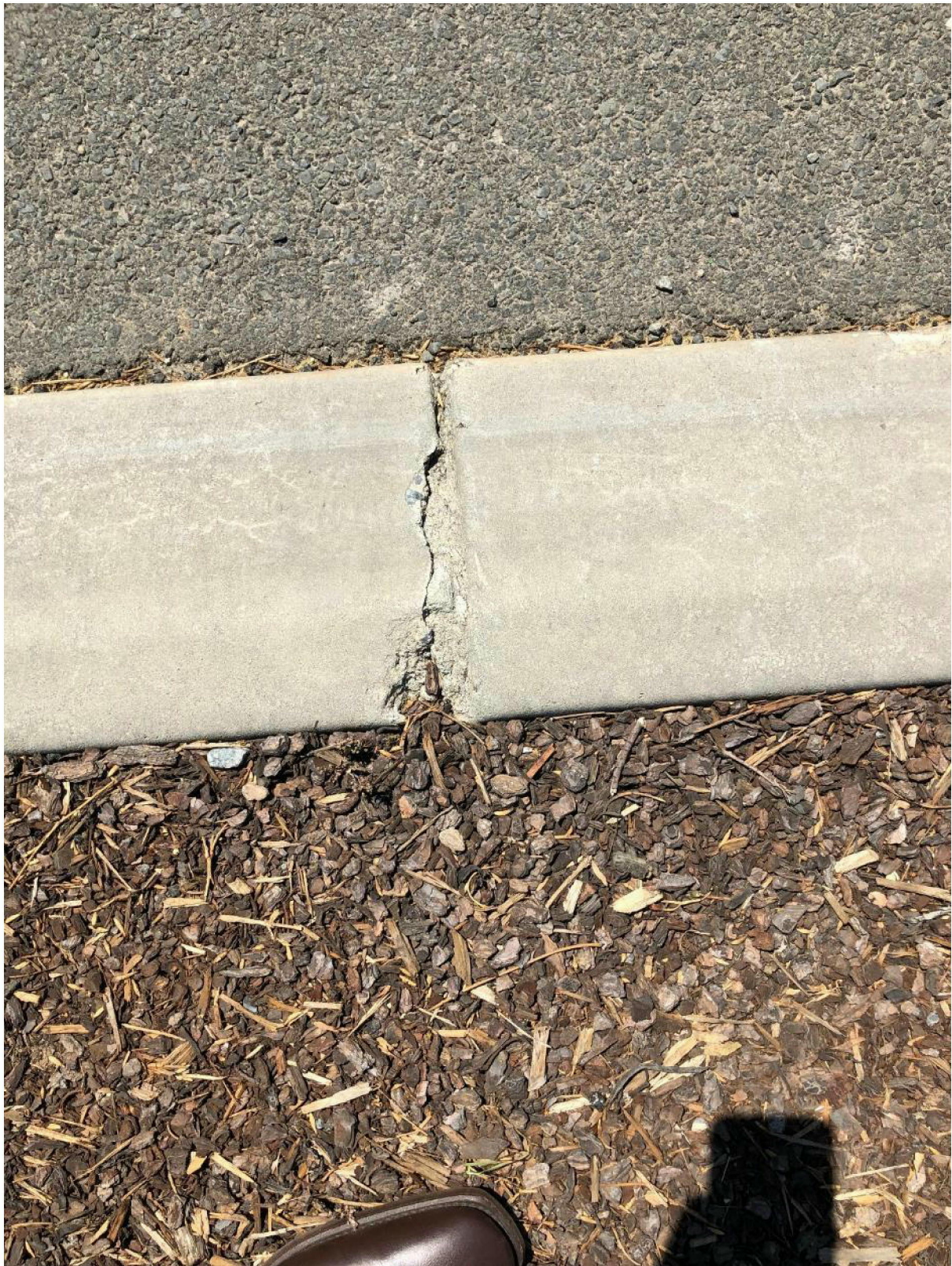
Figure 16: cracking on construction joint interface.
