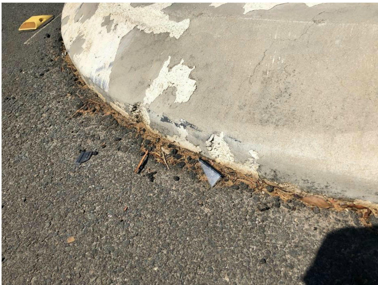
Figure 1: chips in median strip kerb (facing The Northern Road)
