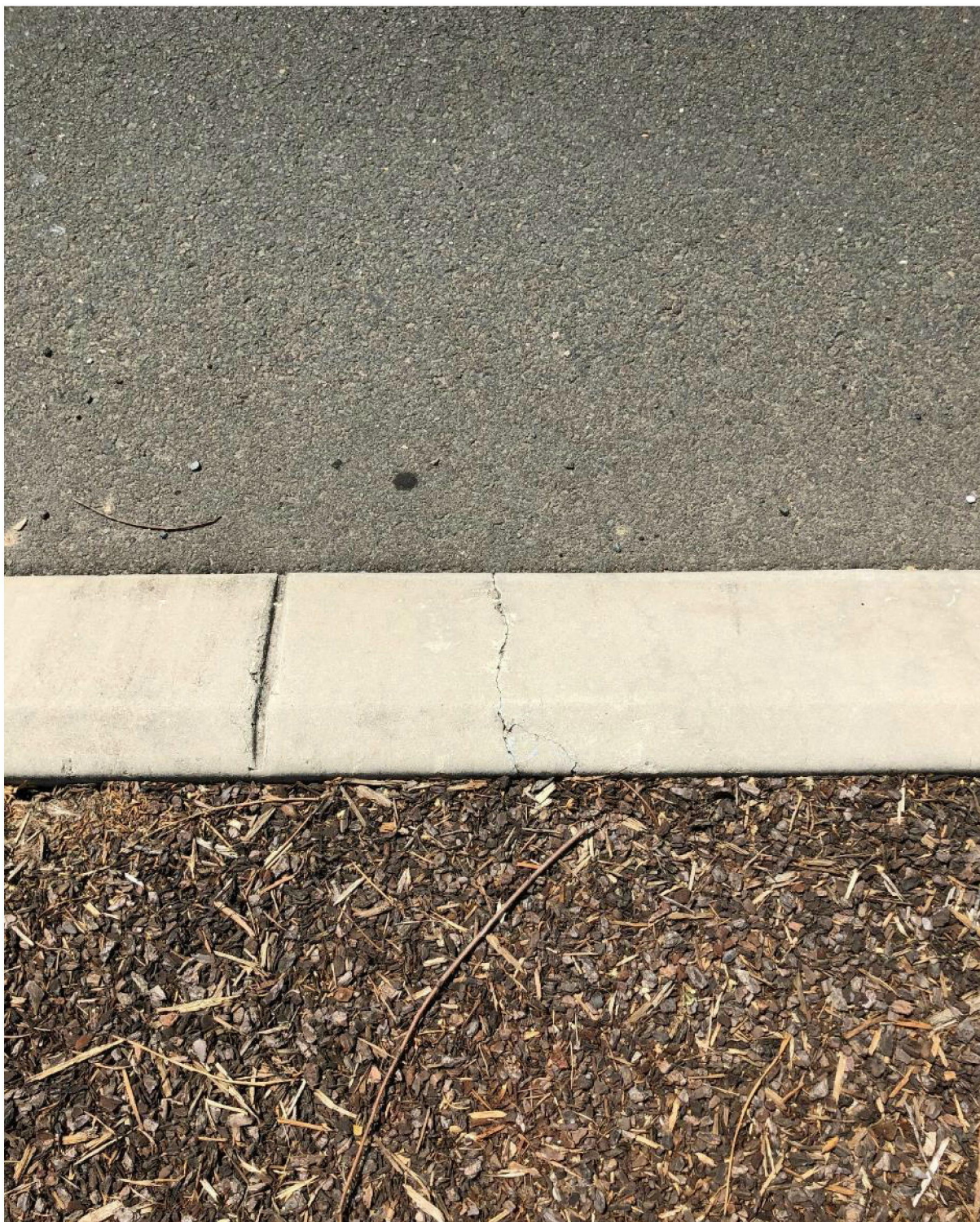
Figure 8: cracking to median strip kerb.
