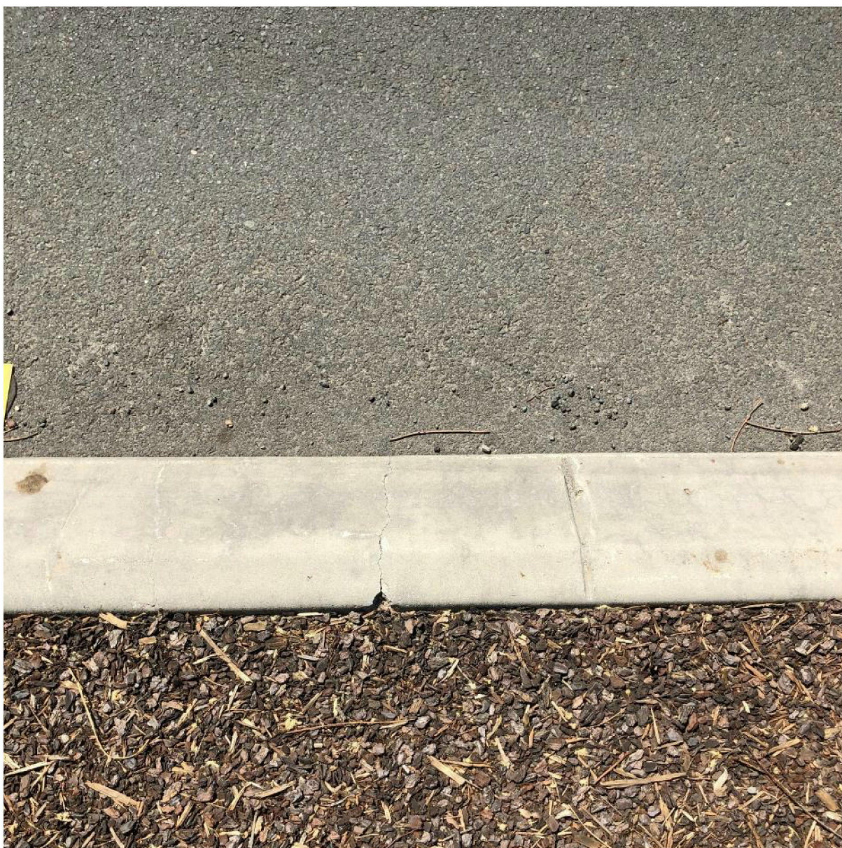
Figure 9: cracking to median strip kerb.
