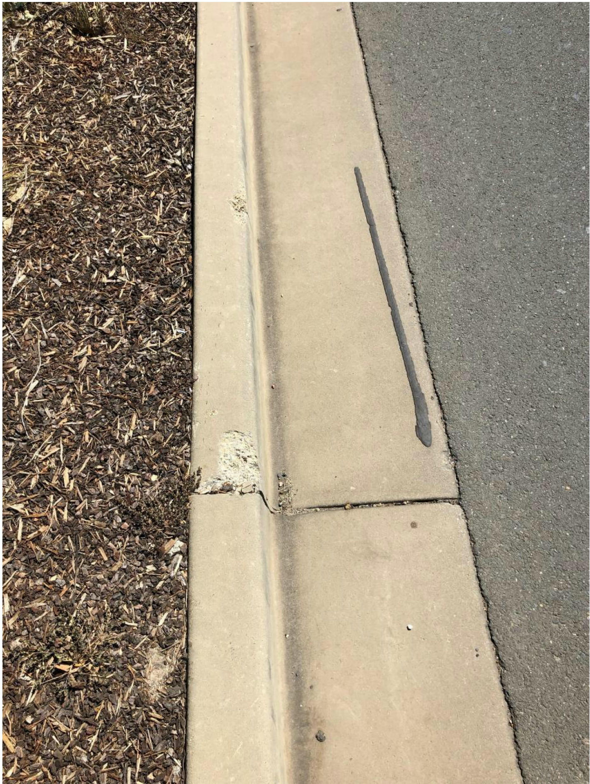
Figure 61: chip to top of kerb. Crack seal residue on gutter.
