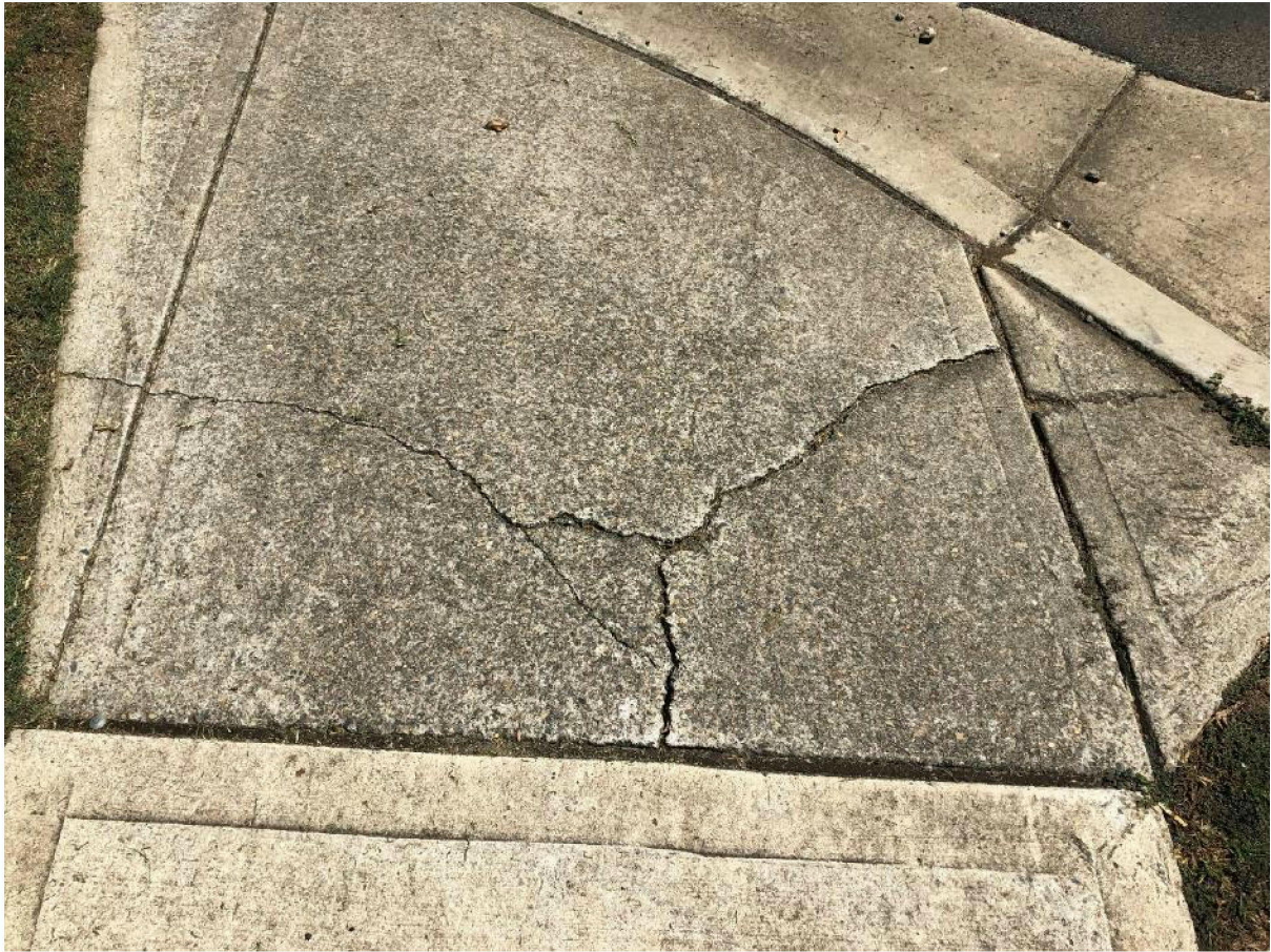
Figure 85: cracking to pram ramp located left of proposed site entry.
