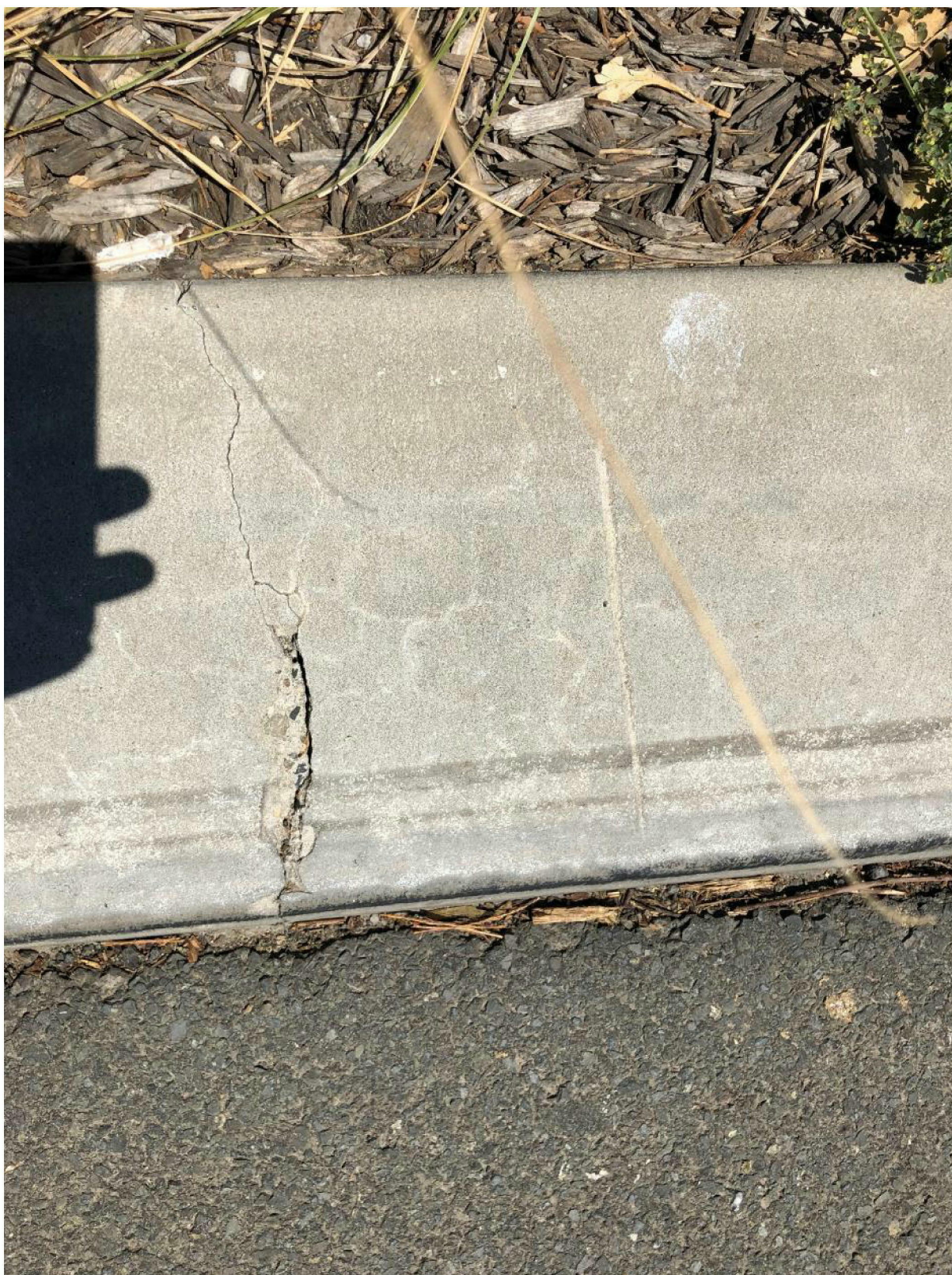
Figure 24: cracking to median strip kerb.
