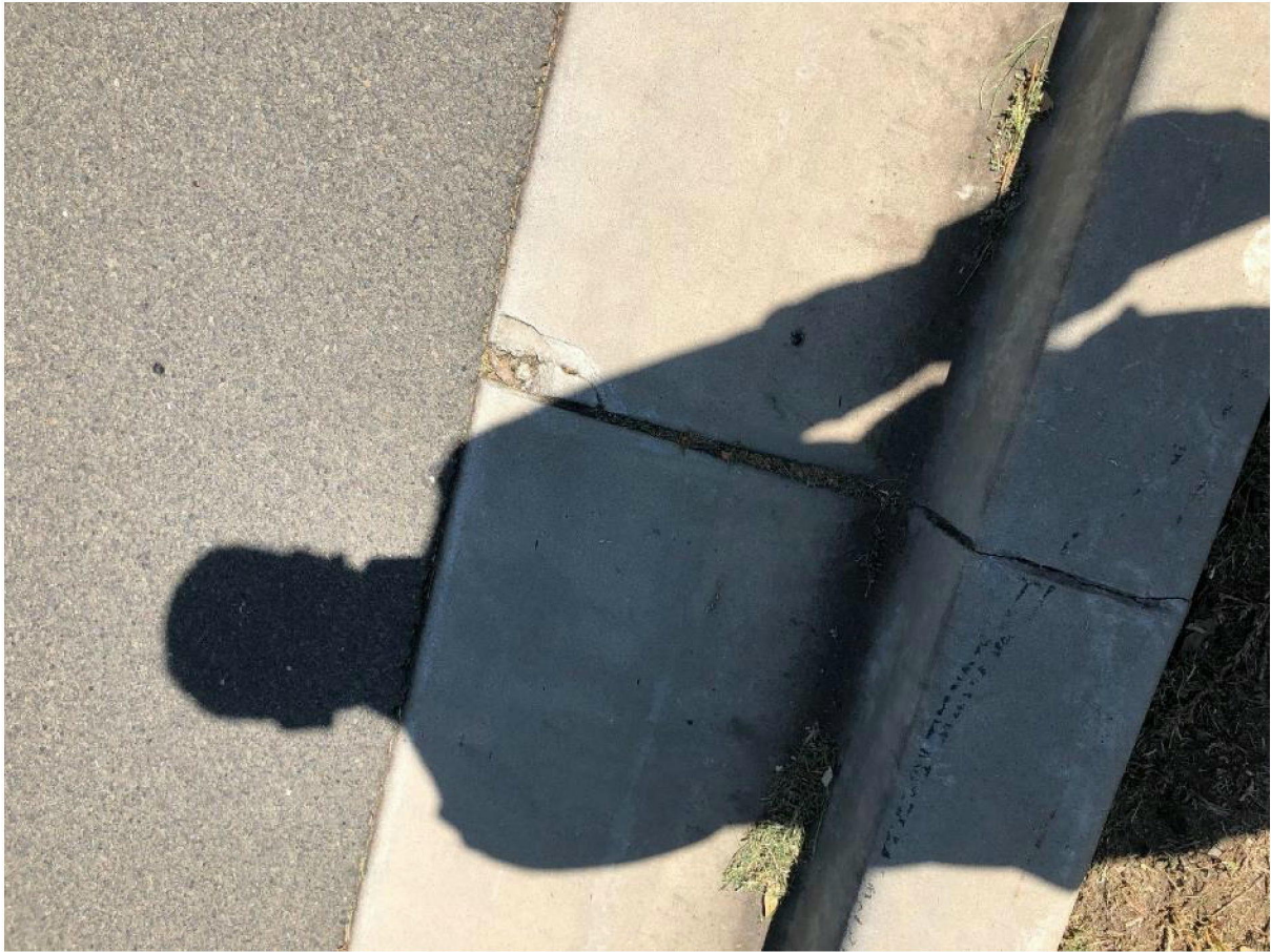
Figure 72: chip to gutter at construction joint interface.
