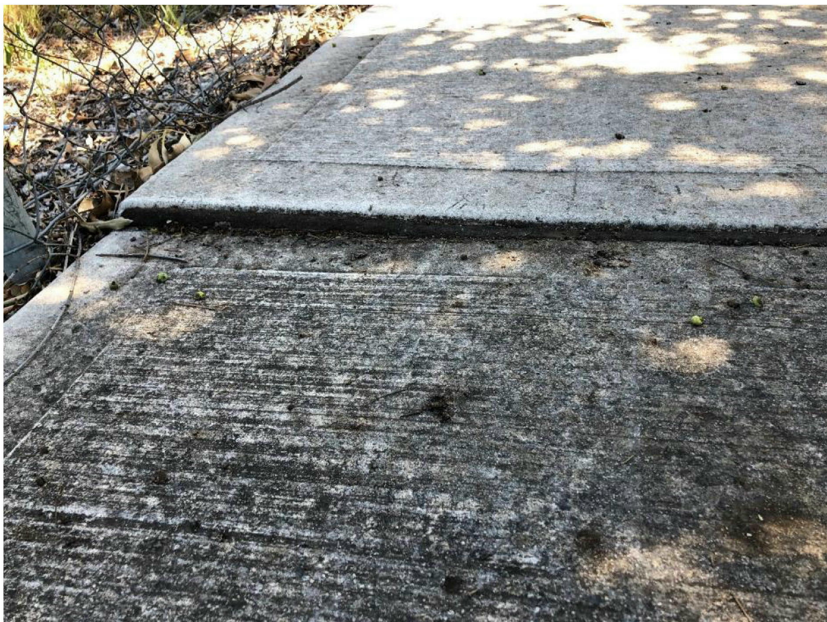
Figure 87: footpath bay lifted at expansion joint interface.
