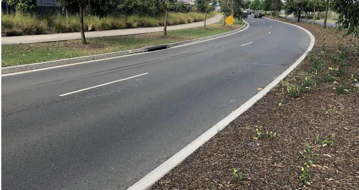
Figure 88: Approx CH250 EB pavement failure (P53)
