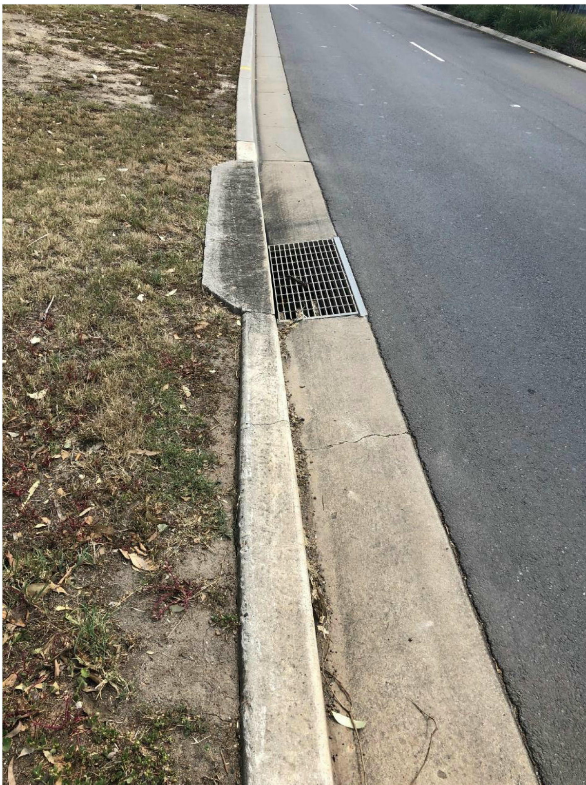
Figure 49: cracking on kerb and gutter, adjacent to SW pit.
