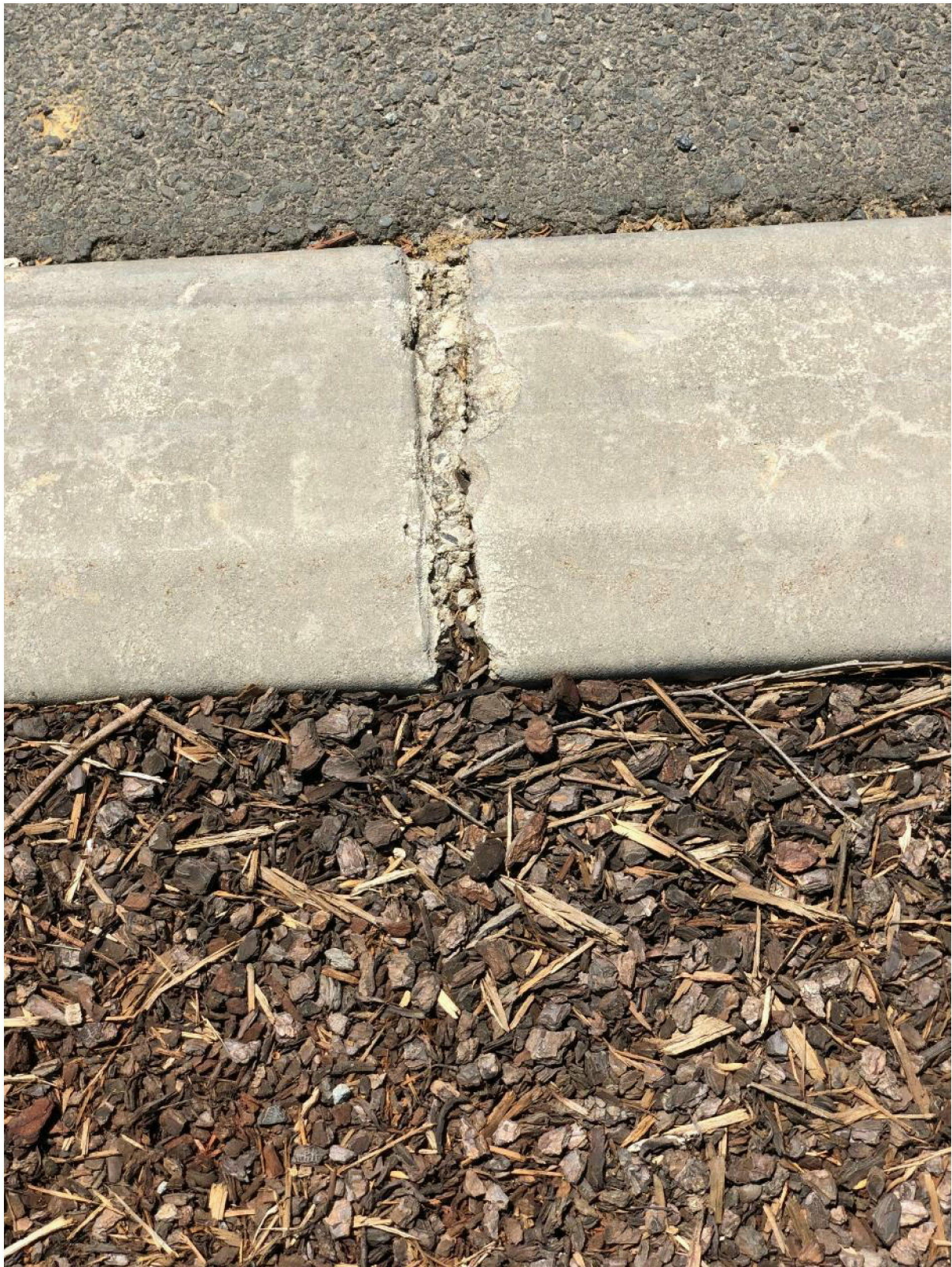
Figure 18: separation of median strip kerb.
