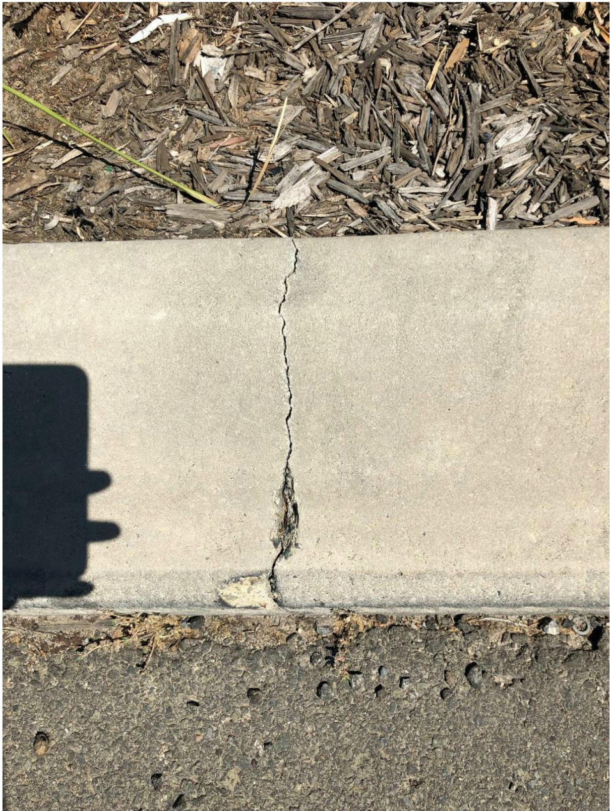
Figure 4: crack in median strip kerb.
