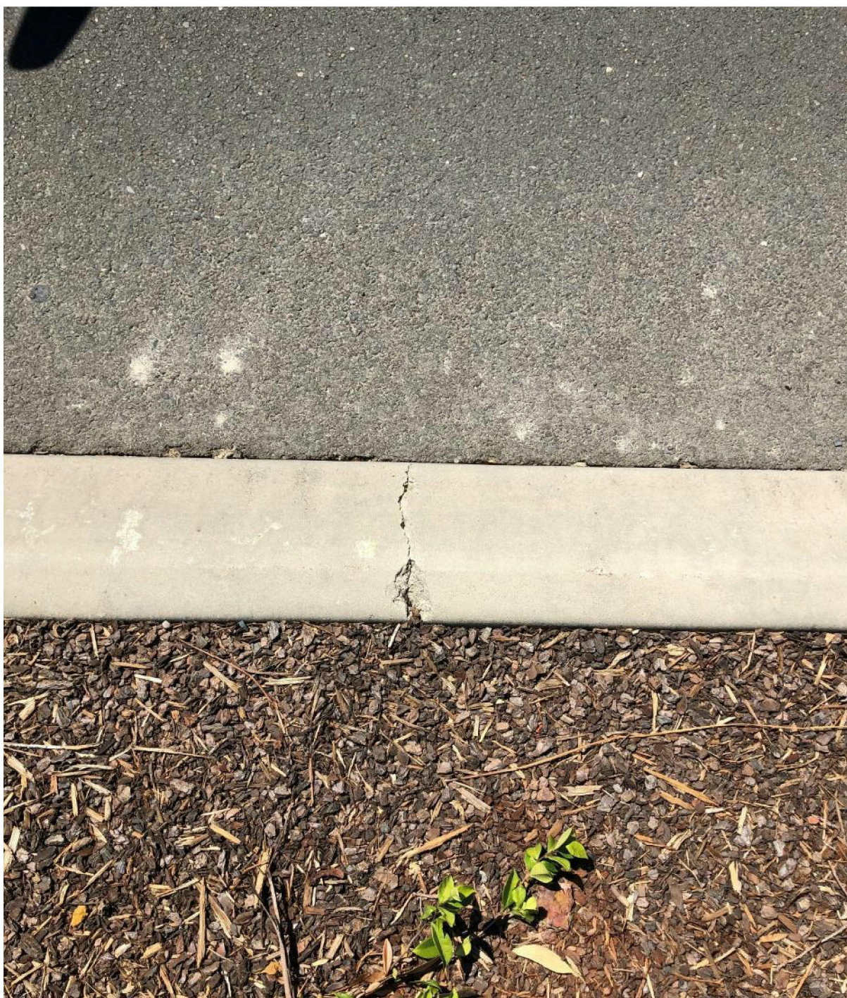
Figure 6: cracking to median strip kerb.
