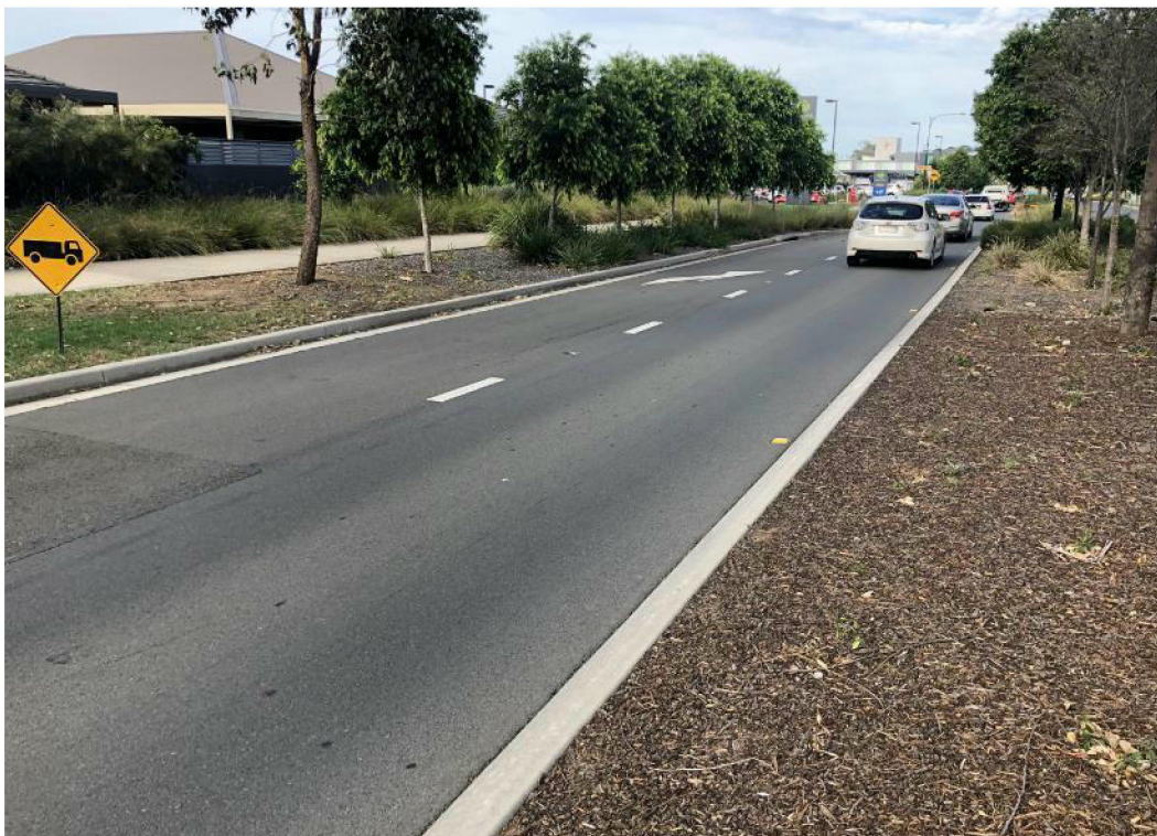
Figure 91: Approx CH320 EB Pavement failure
