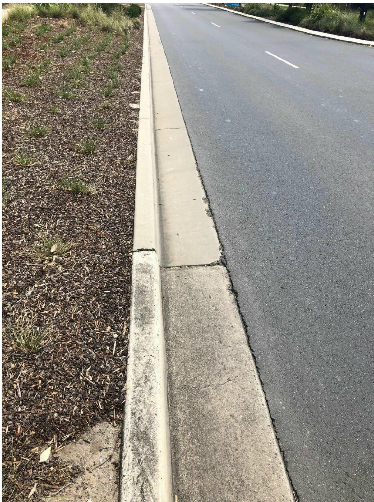
Figure 59: chip to gutter and cracking to kerb and gutter.
