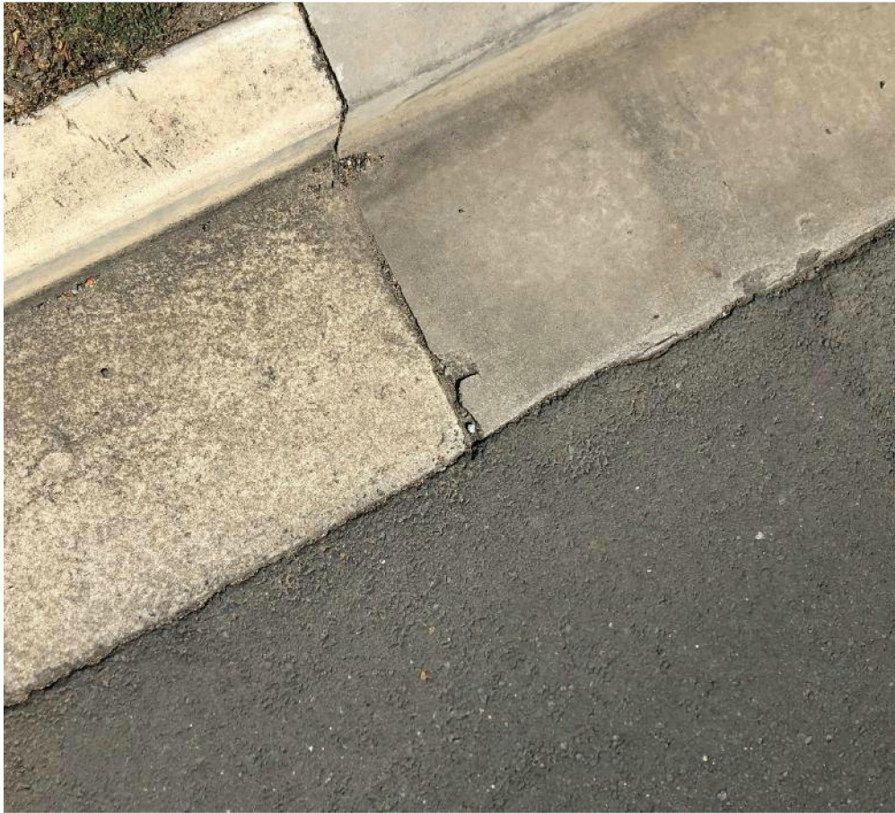
Figure 42: spalling on edge of construction joint interface on gutter.
