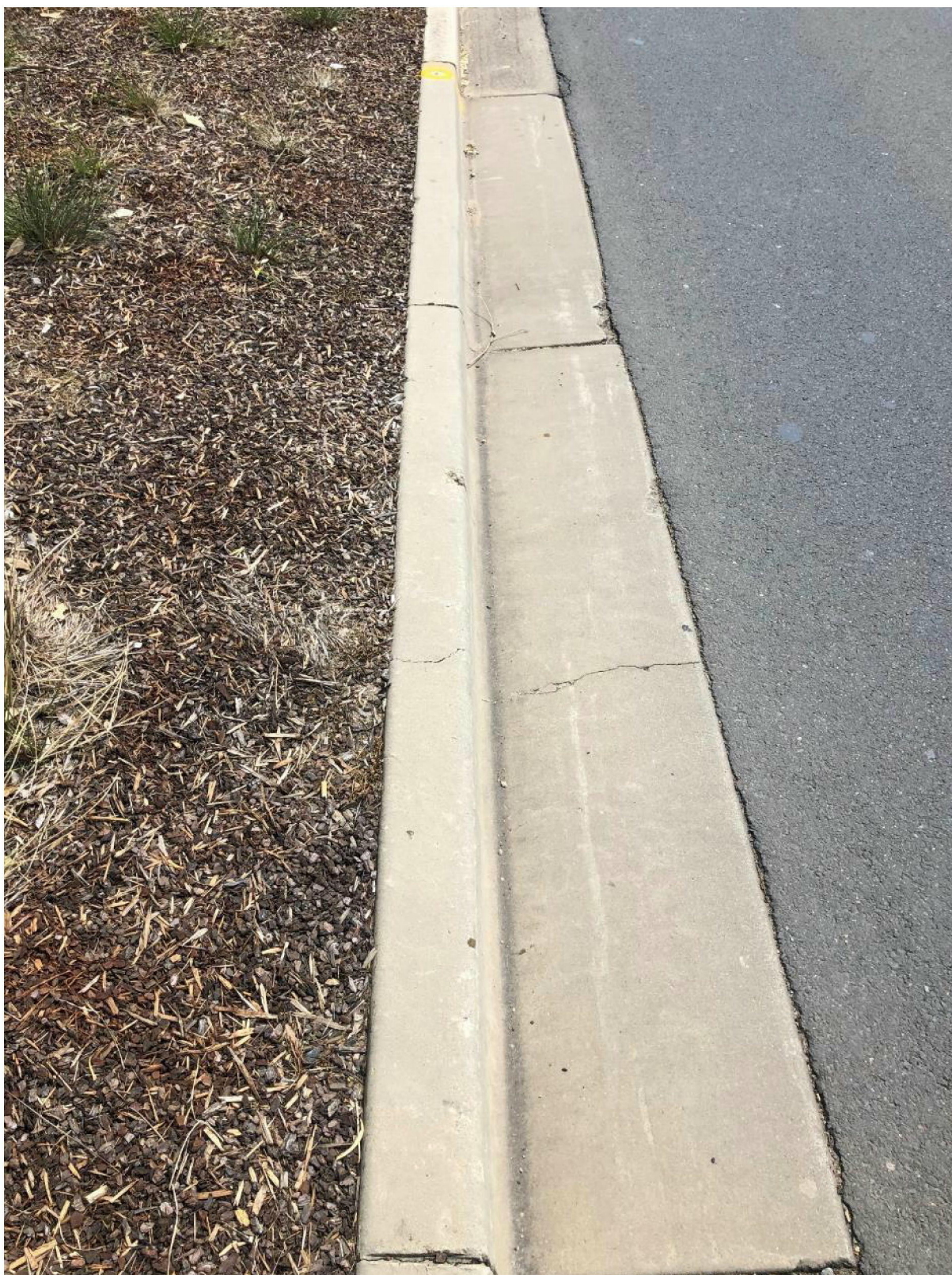
Figure 57: cracking on kerb and gutter as well as chips to gutter.
