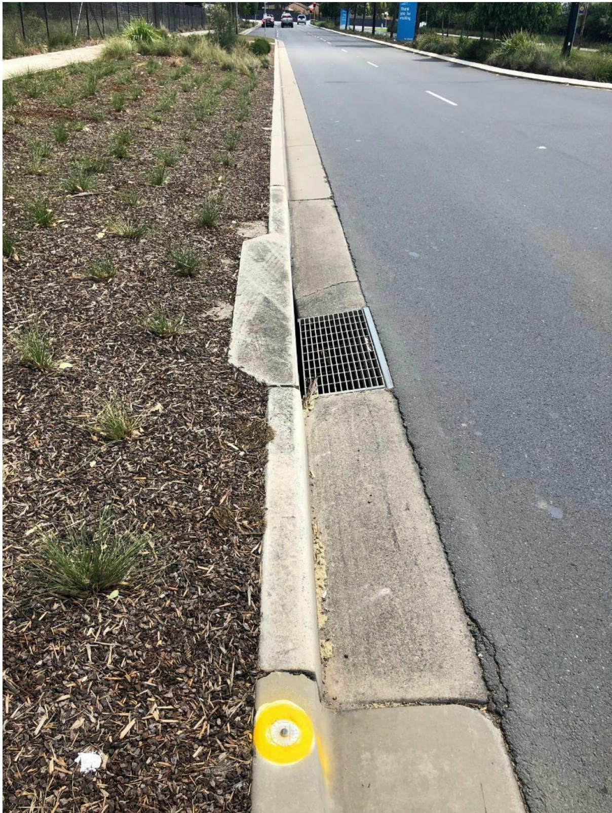
Figure 58: damage to asphalt (adjacent to expansion joint), cracking to gutter (adjacent to SW pit) and damage to top of gutter (expansion joint interface).
