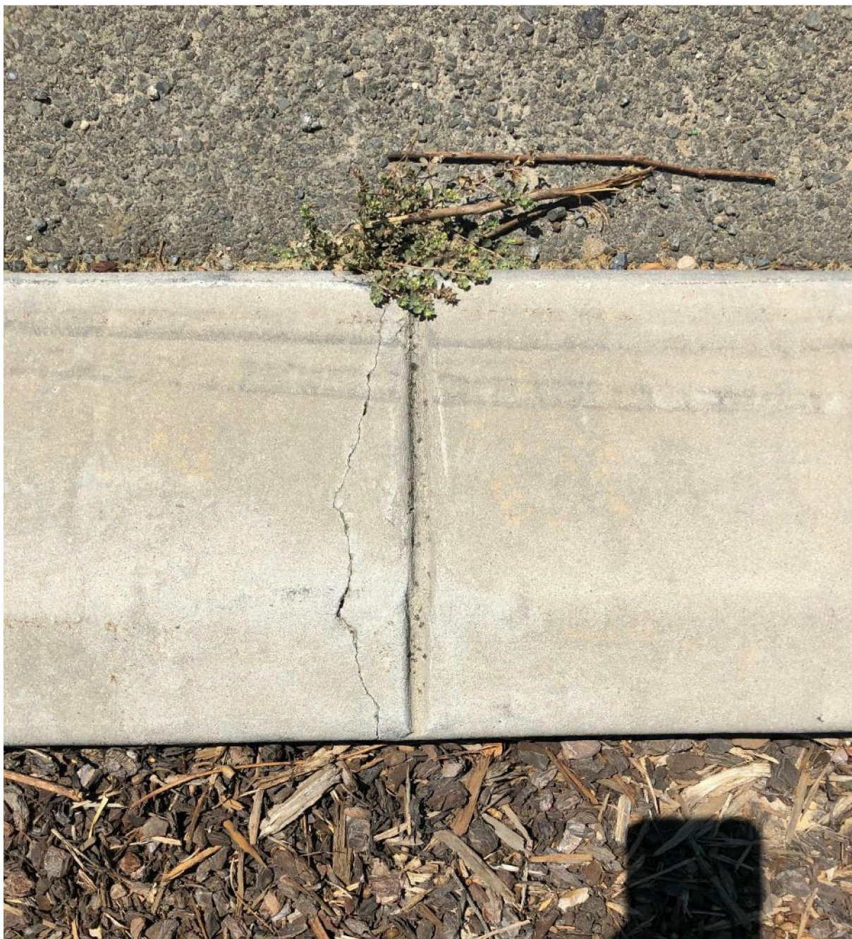
Figure 13: cracking to median strip kerb.
