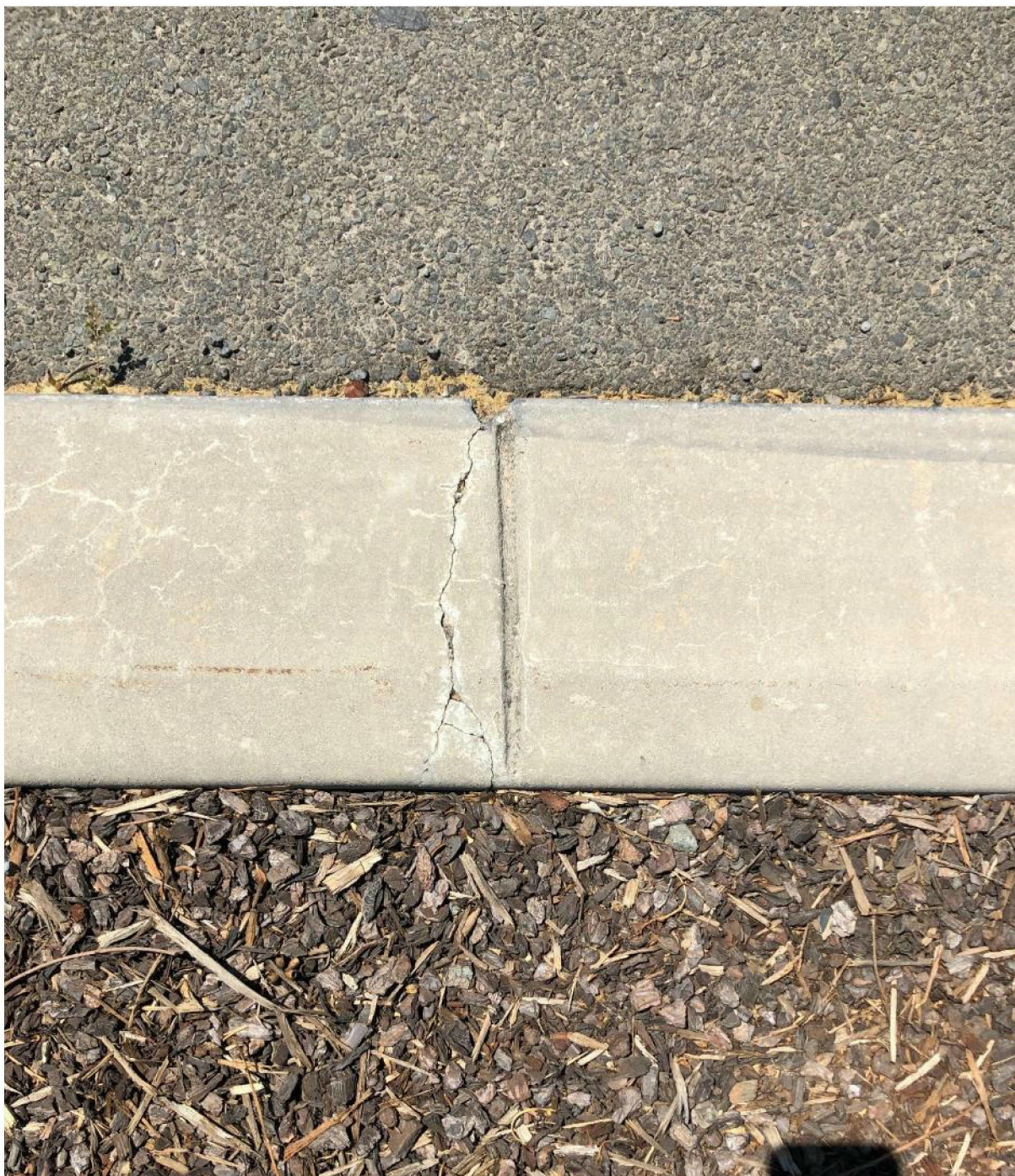
Figure 14: cracking to median strip kerb.
