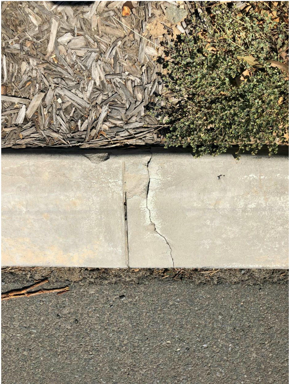
Figure 25: cracking to median strip kerb.
