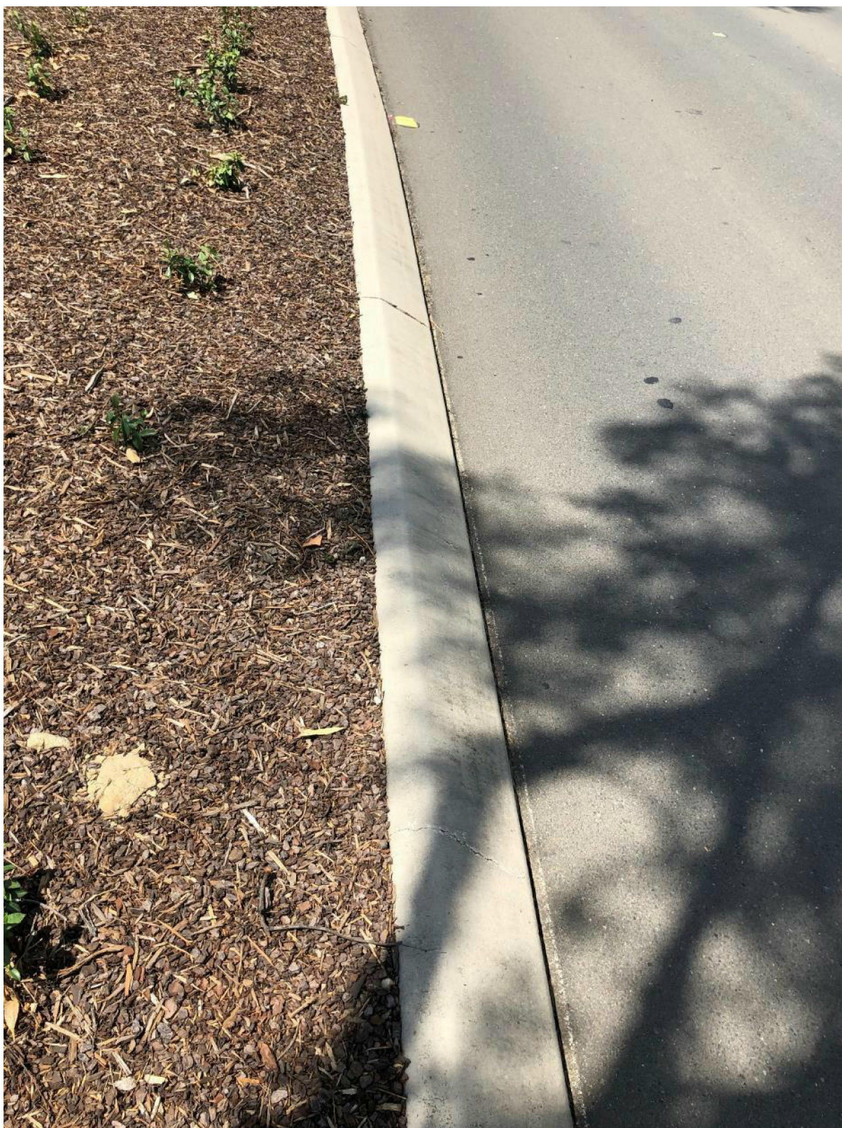
Figure 37: cracking to median strip kerb.
