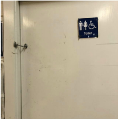
Signage to Accessible toilet
