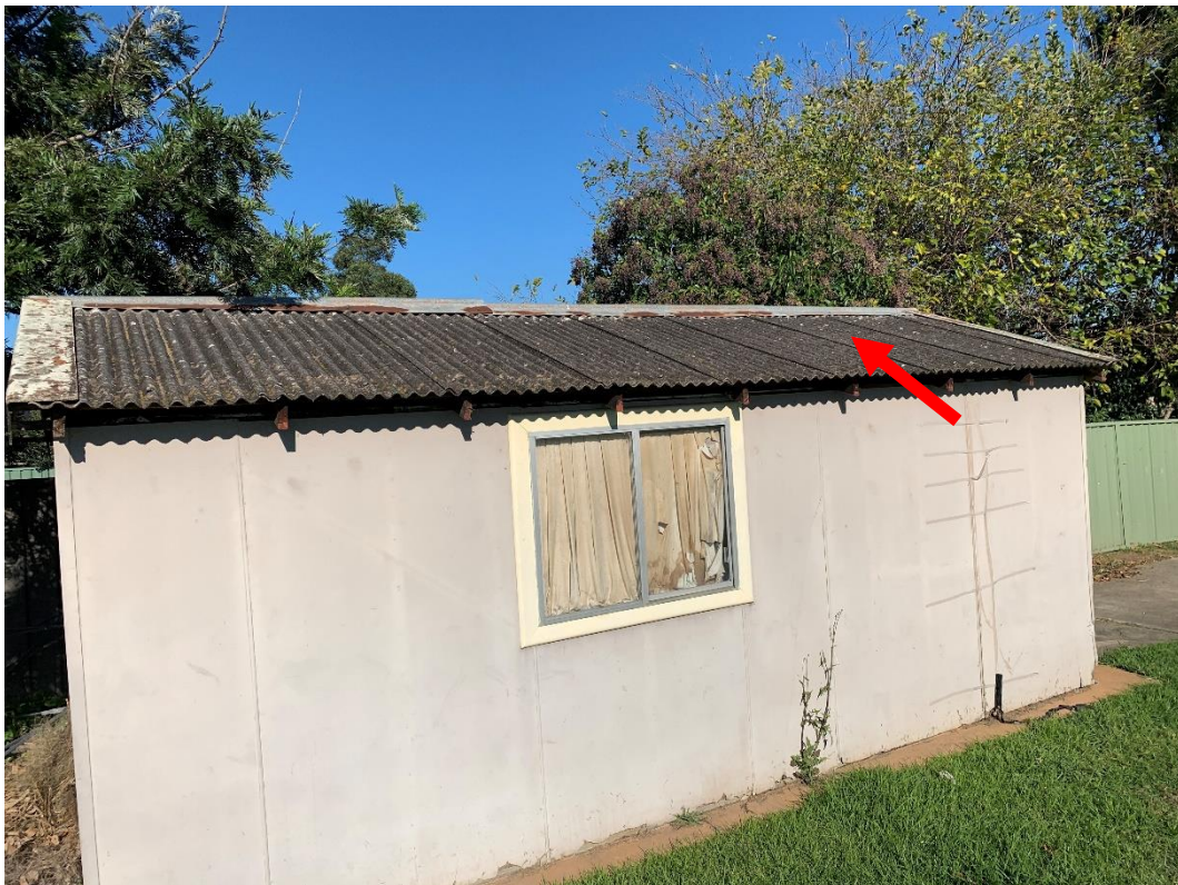
Photo 6: Showing rear garage roof of 40 Mamre Road, St Marys, contains ACM.
