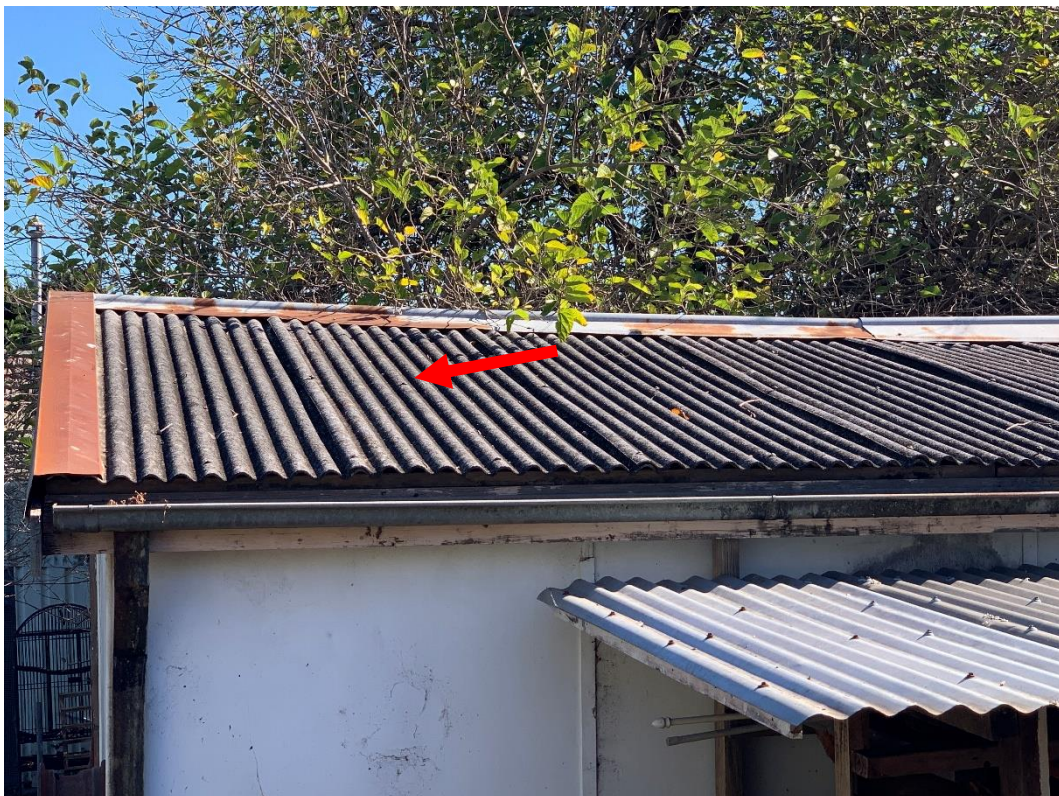
Photo 24: Showing exterior roof of garage at 42 Mamre Road, St Marys NSW, contains ACM.
