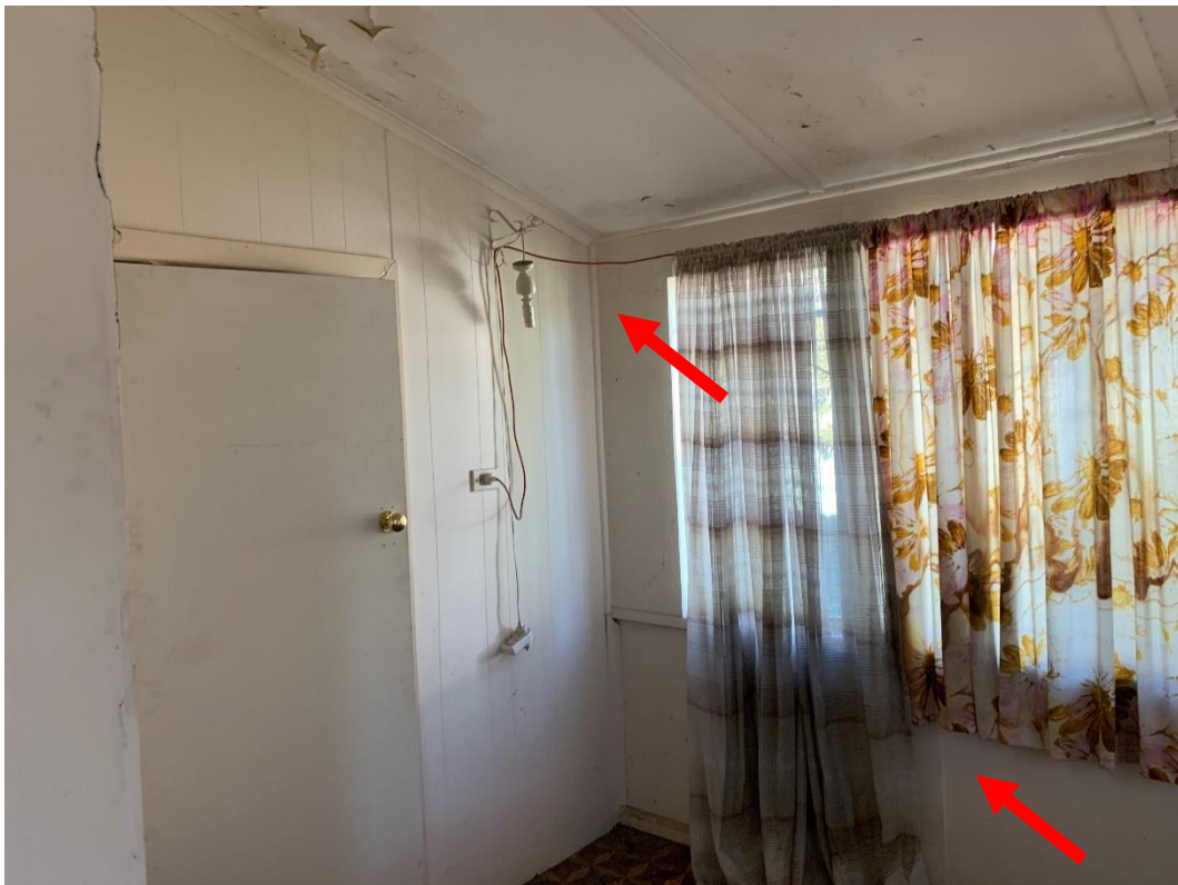
Photo 20: Showing front sunroom walls at 42 Mamre Road, St Marys NSW, contains ACM.
