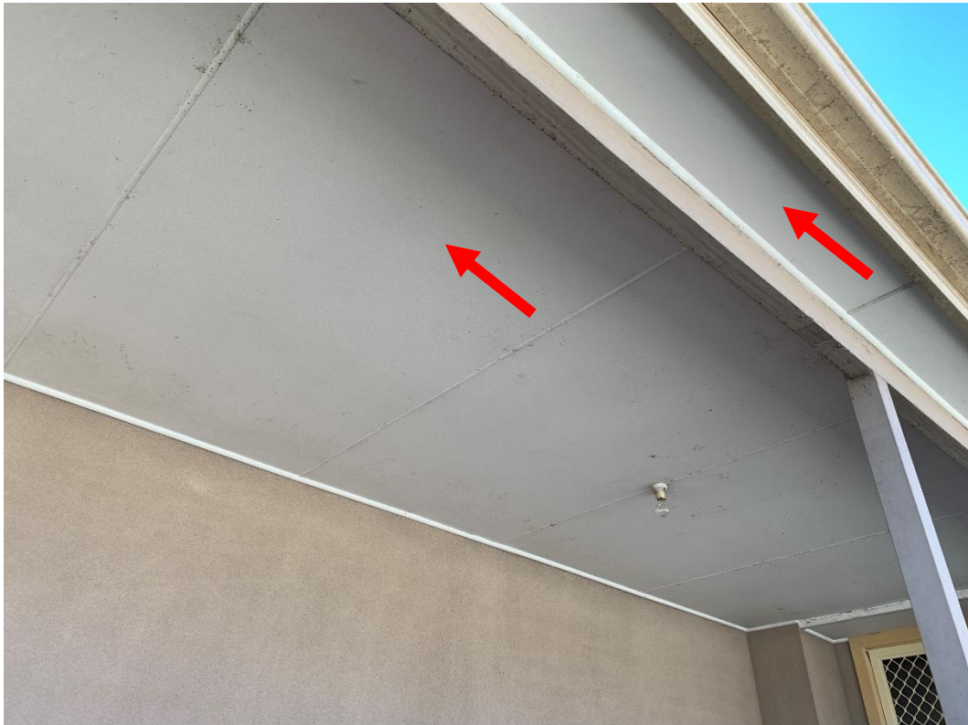
Photo 4: Showing exterior perimeter eaves of 40 Mamre Road, St Marys, contains ACM.
