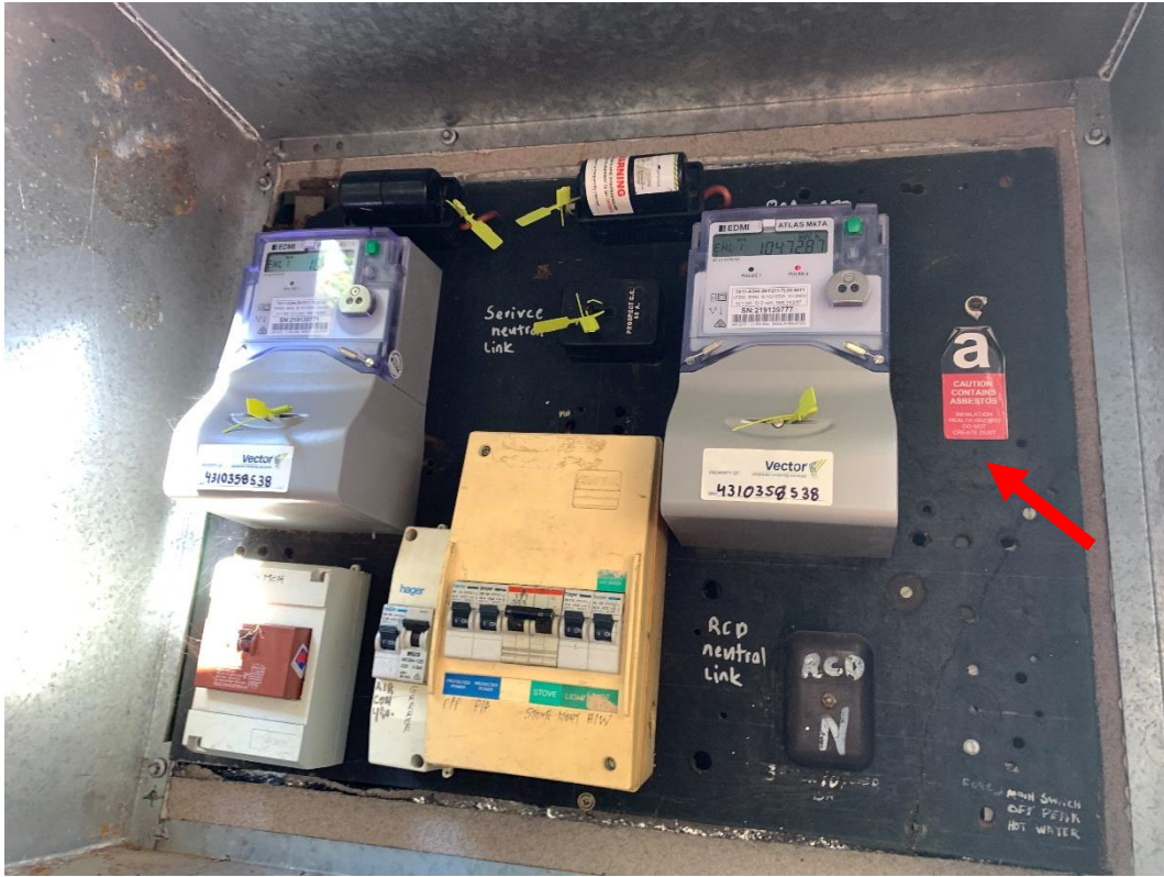
Photo 3: Showing electrical meter backing boards of 40 Mamre Road, S Marys, contains ACM.
