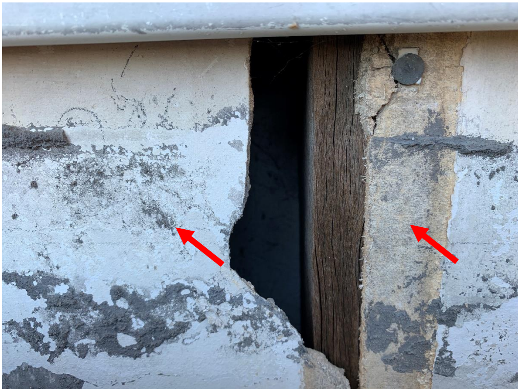
Photo 12: Showing external walls beneath existing cladding at 42 Mamre Road, St Marys NSW, contains ACM.
