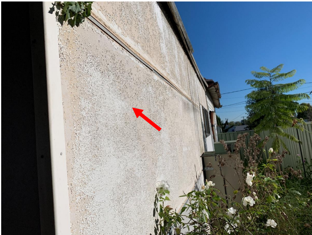
Photo 22: Showing exterior side walls at 42 Mamre Road, St Marys NSW, contains ACM.
