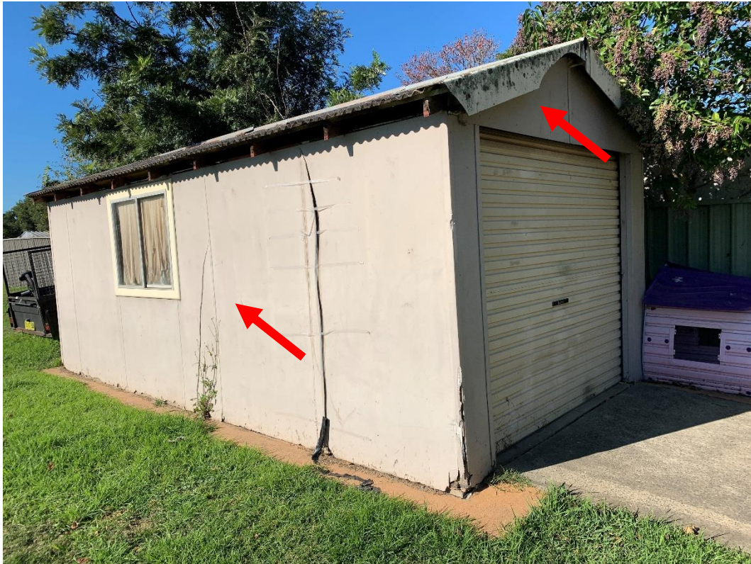
Photo 5: Showing rear garage walls of 40 Mamre Road, St Marys, contains ACM.
