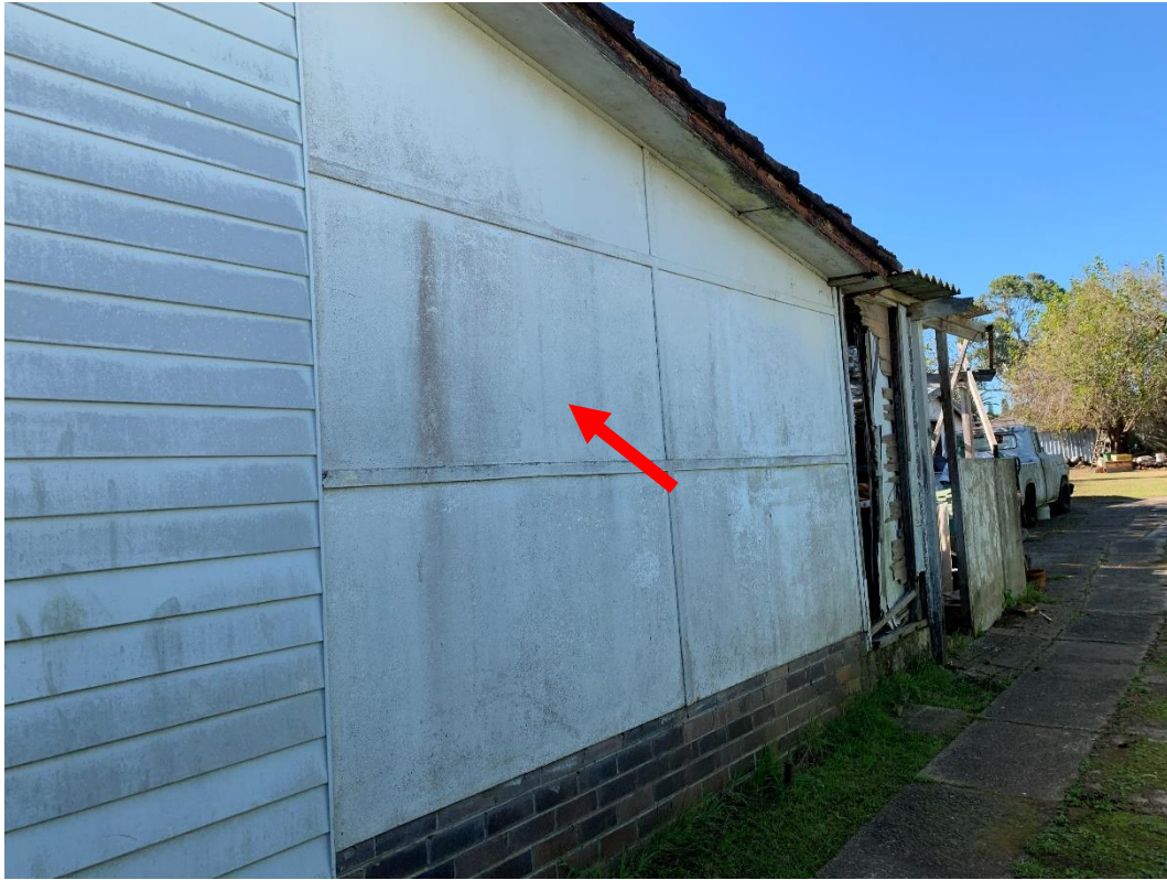
Photo 13: Showing external rear walls at 42 Mamre Road, St Marys NSW, contains ACM.
