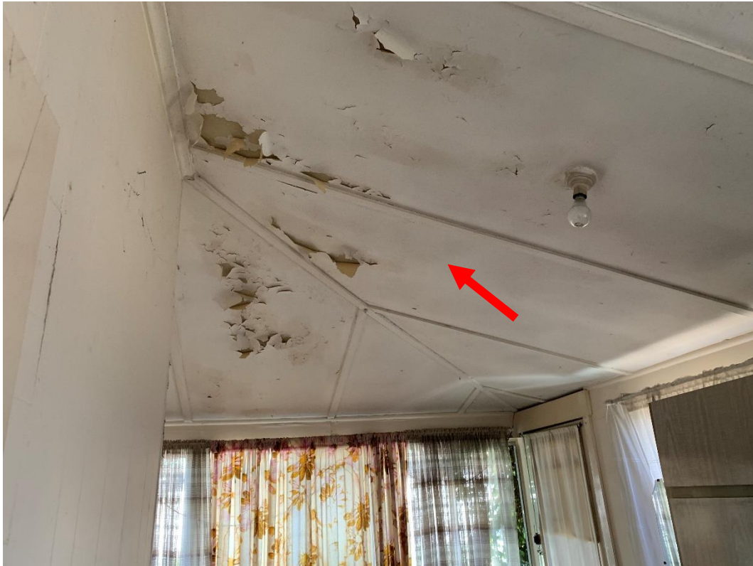
Photo 19: Showing front sunroom ceiling at 42 Mamre Road, St Marys NSW, contains ACM.
