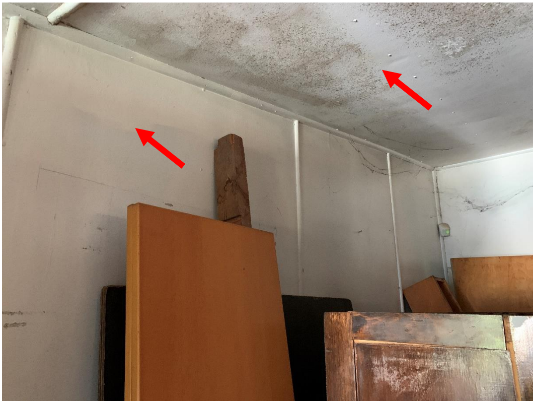
Photo 16: Showing interior dining walls and ceiling at 42 Mamre Road, St Marys NSW, contains ACM.
