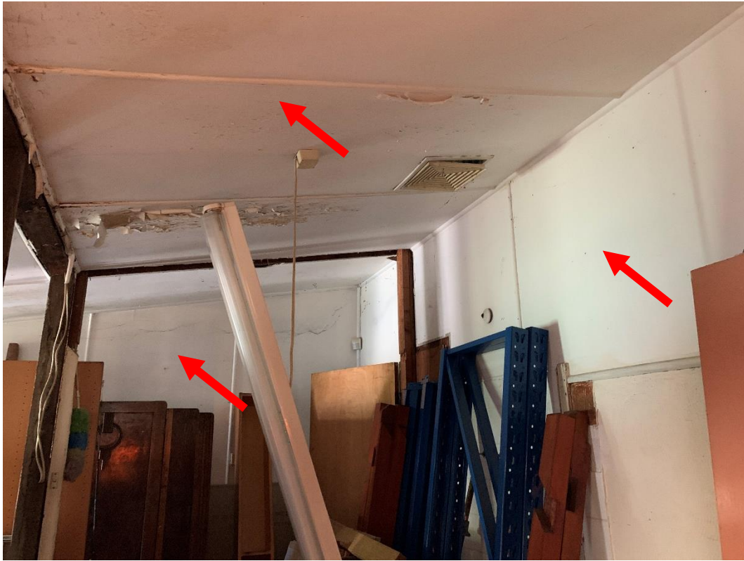
Photo 21: Showing front bedroom walls and ceiling at 42 Mamre Road, St Marys NSW, contains ACM.
