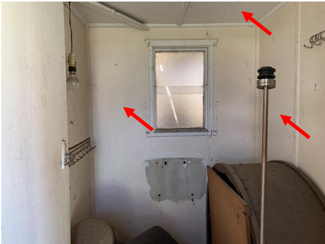
Photo 14: Showing interior toilet walls and ceiling at 42 Mamre Road, St Marys NSW, contains ACM.
