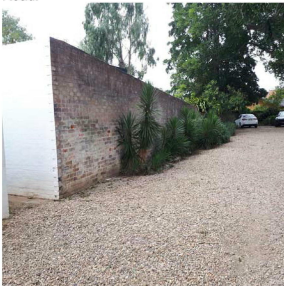
Carpark South east view – Succulents on western face of common wall with Lewers Courtyard.
