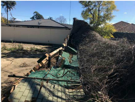
Photograph: South west corner of boundary Western section - Collapse face brick boundary wall
