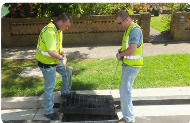
Photo 9 Lift grate above the support frame
