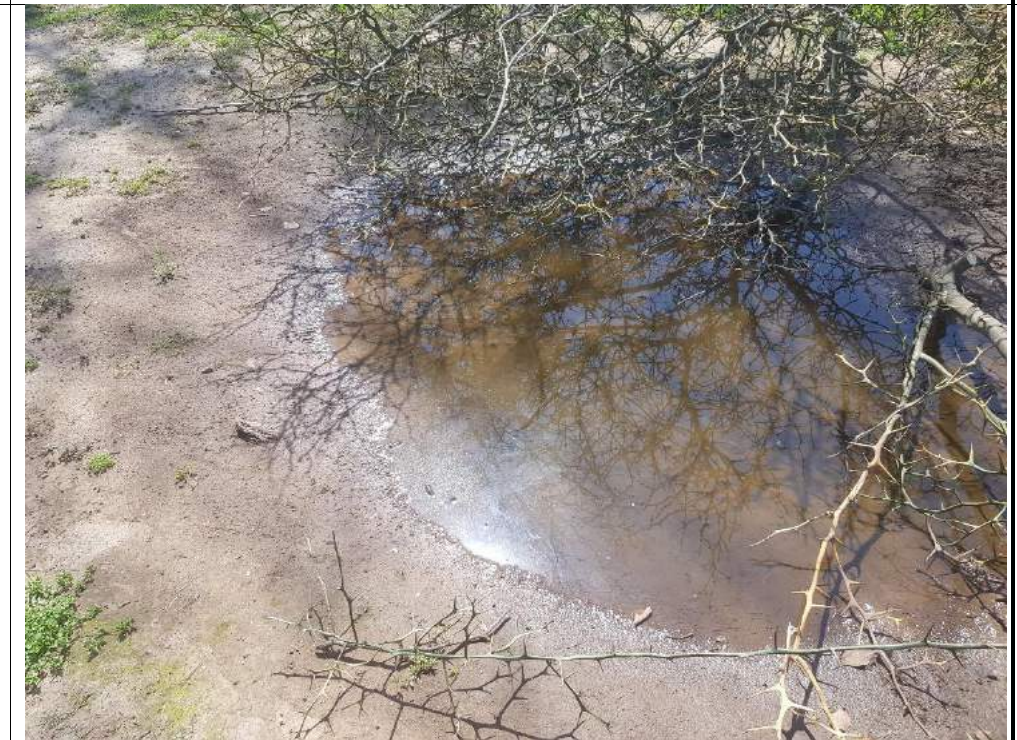
Photograph 6 – Rain water pond on vehicle turn around bay, shine on water surface.
