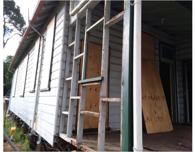
Notes: Overview of the removal item (walls panels to the southern entrance) following removal
