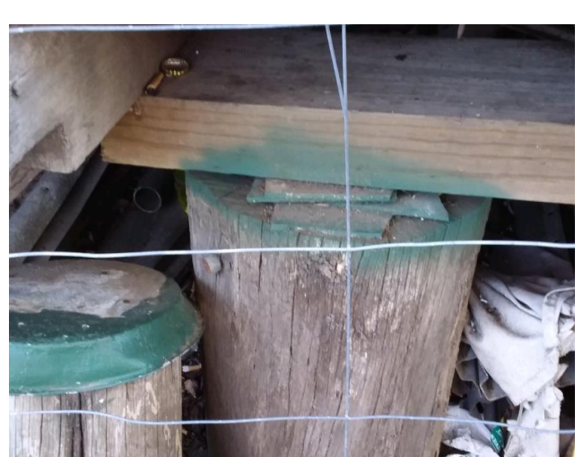
Notes: Condition of packing material
