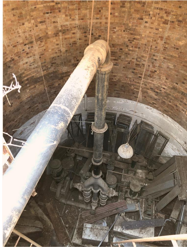
Figure 12 – Interior of the remnant Pump House. Showing the internal pumping equipment.
