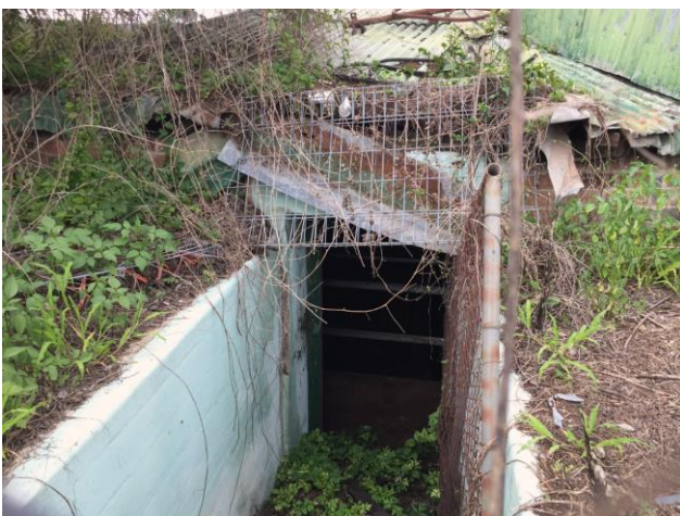
Figure 19 – Entrance to the remnant Pump House (from Lot 21) lies below grade with steps into the entry.
