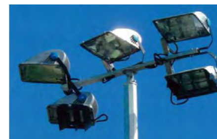
TYPICAL NETBALL AND BASKETBALL COURT LIGHTING LUMINAIRE ARRANGEMENT. INDICATIVE ONLY. FINAL LUMINAIRE TYPES AND QUANTITIES PER POLE TO BE CONFIRMED
